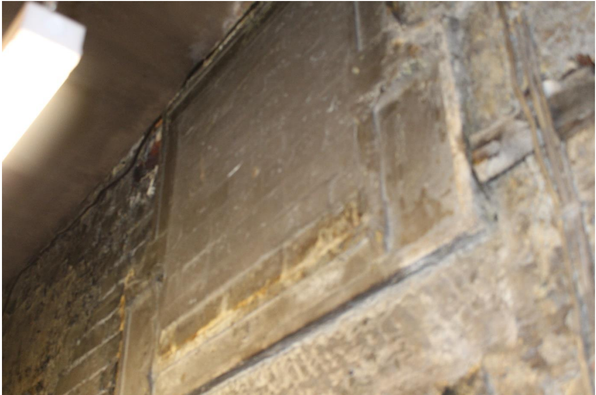
Plate 30 – Boiler House Drive Shaft
