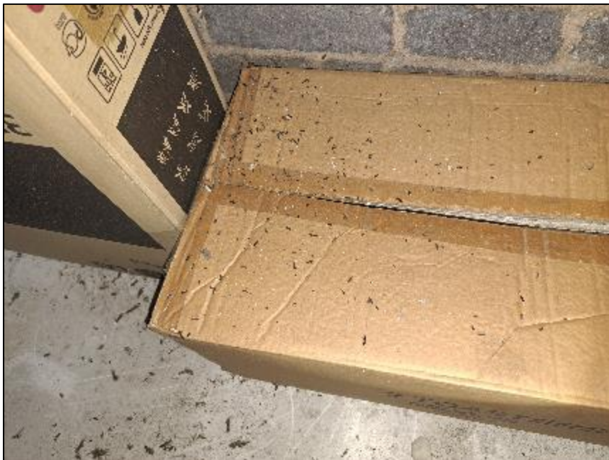
Photograph 8. Showing the accumulation of bat droppings found within the roof void
