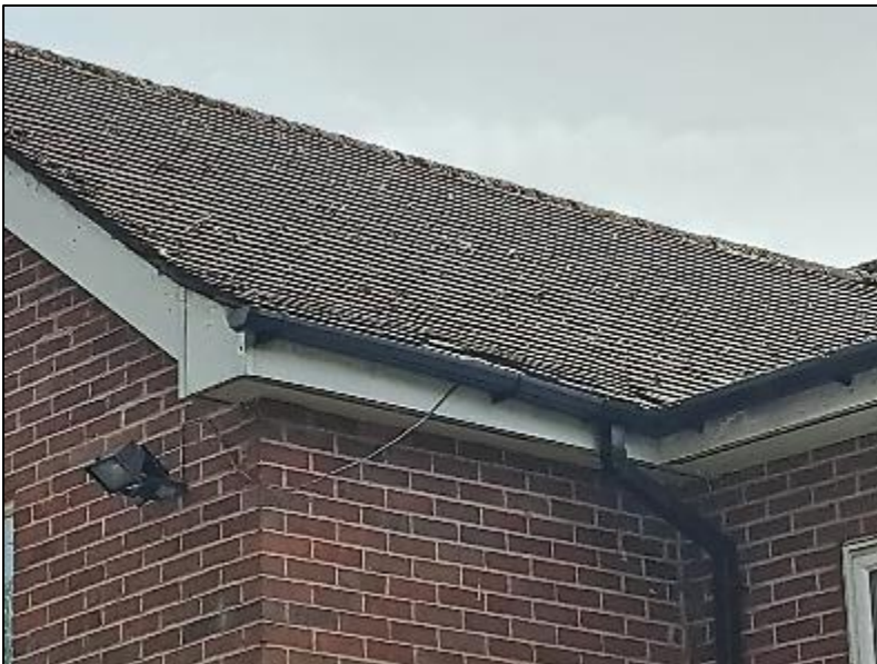
Photograph 3. Showing some missing tiles at the front of the building
