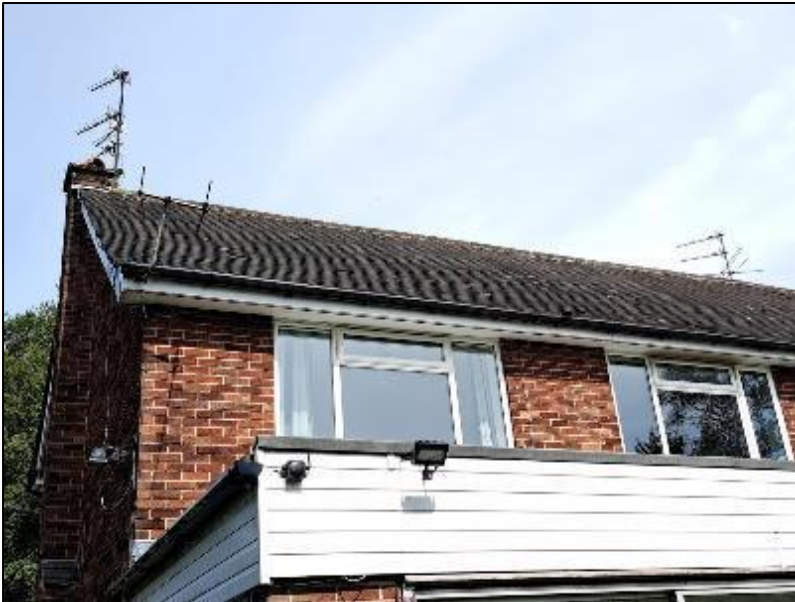
Photograph 2. Showing the slipped and missing tiles at the rear of the building
