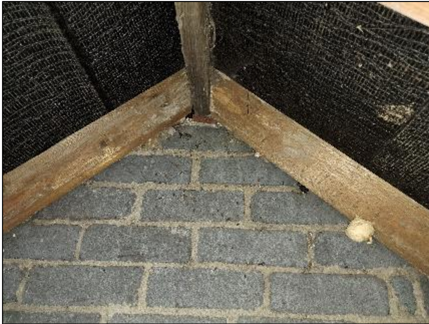
Photograph 7. Showing the gap in the brickwork above the accumulation of bat droppings
