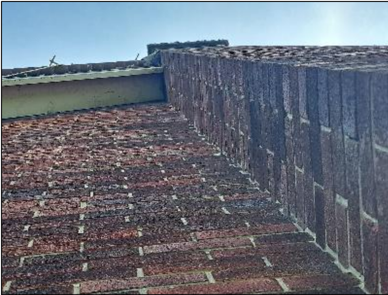
Photograph 4. Showing gapping between soffit boards and chimney breast on the western gable
