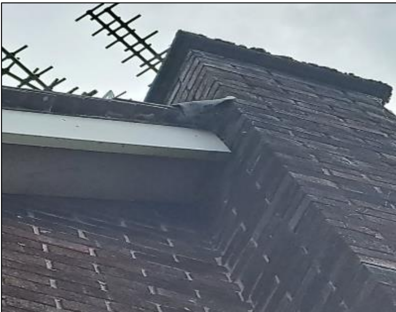
Photograph 5. Showing lifted flashing at one of the gable ends
