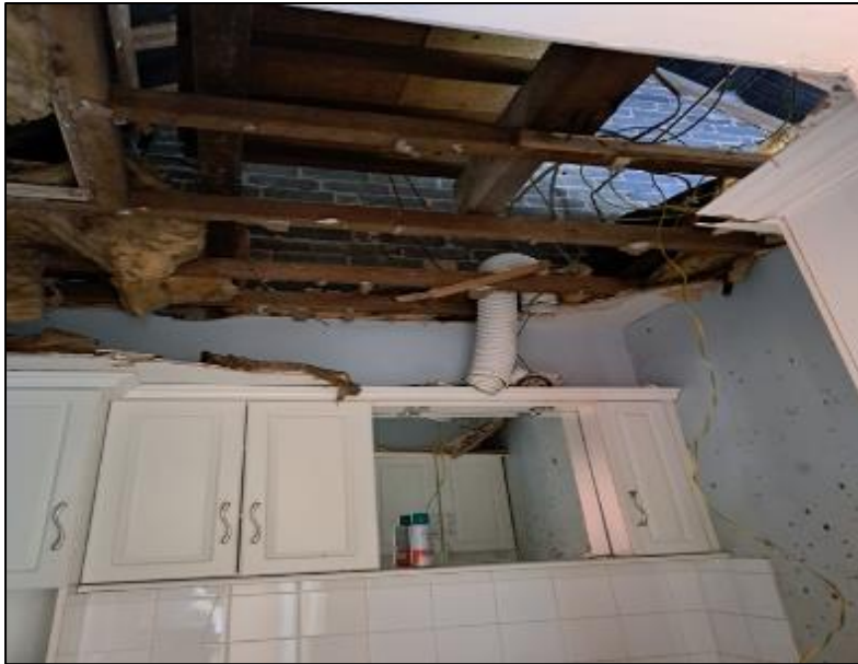
Photograph 6. Showing where the ceiling had collapsed, exposing the roof void
