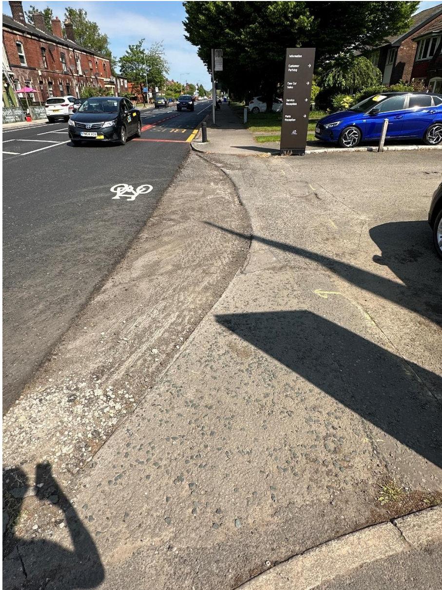
Photo 7 - Unlevelled Surfaces due to Recent Road Improvement Works
