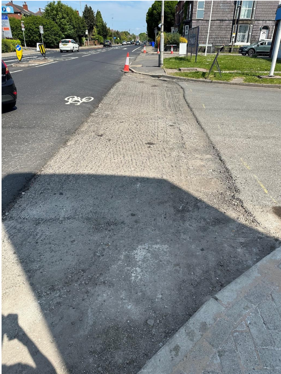
Photo 5 -Unlevelled Surfaces due to Recent Road Improvement Works
