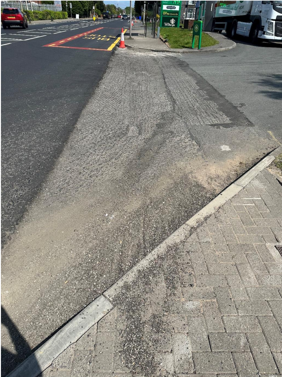
Photo 6 - Unlevelled Surfaces due to Recent Road Improvement Works
