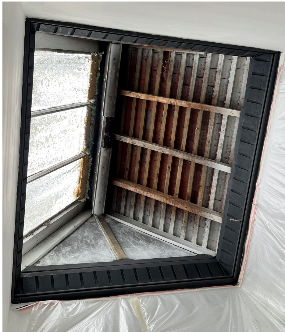
Image: upper floor rooflight, to be reglazed.
