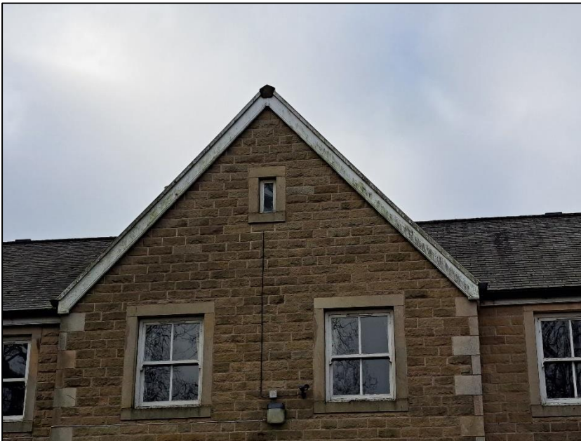
Photograph 6 showing the uPVC barge boards
