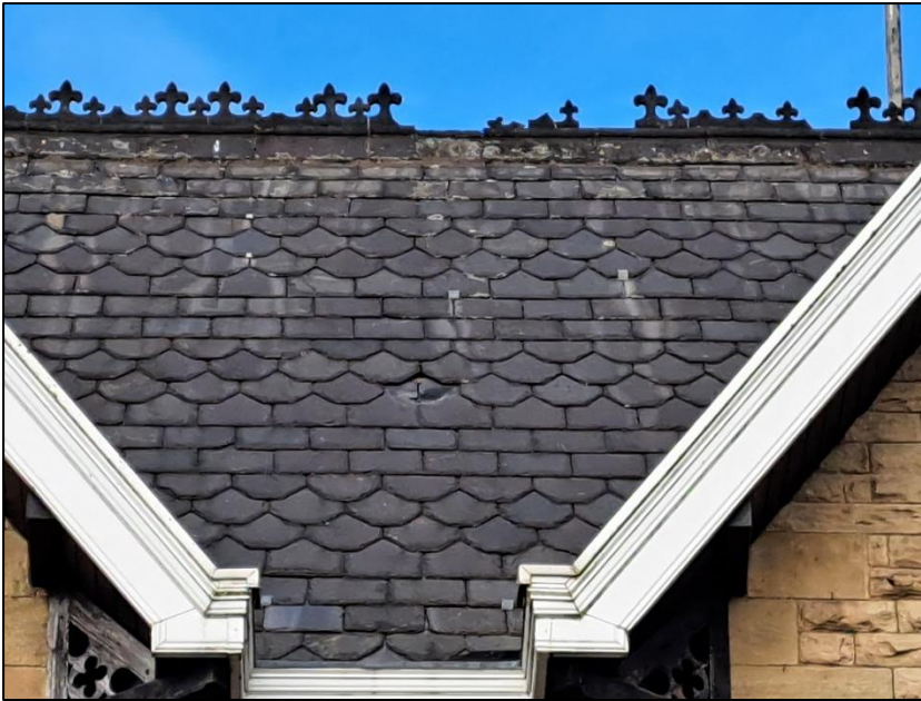
Photograph 5 showing some of the missing roof and ridge tiles
