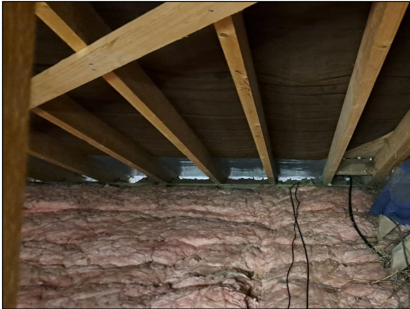
Photograph 11 showing daylight at the roof edges
