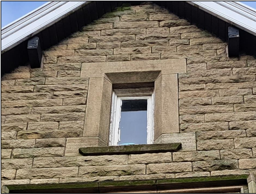
Photograph 3 showing missing mortar
