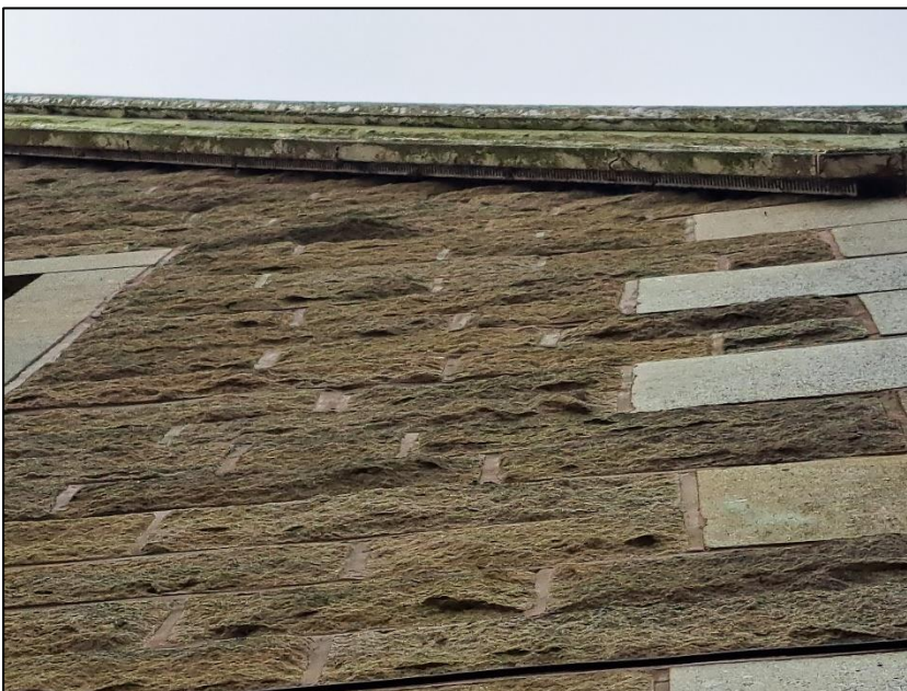
Photograph 8 showing the gaps beneath the barge boards
