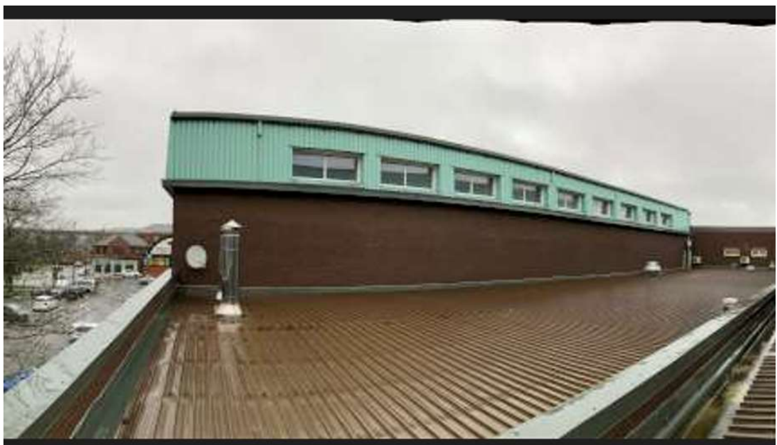
Photograph showing location of both existing and new flues
