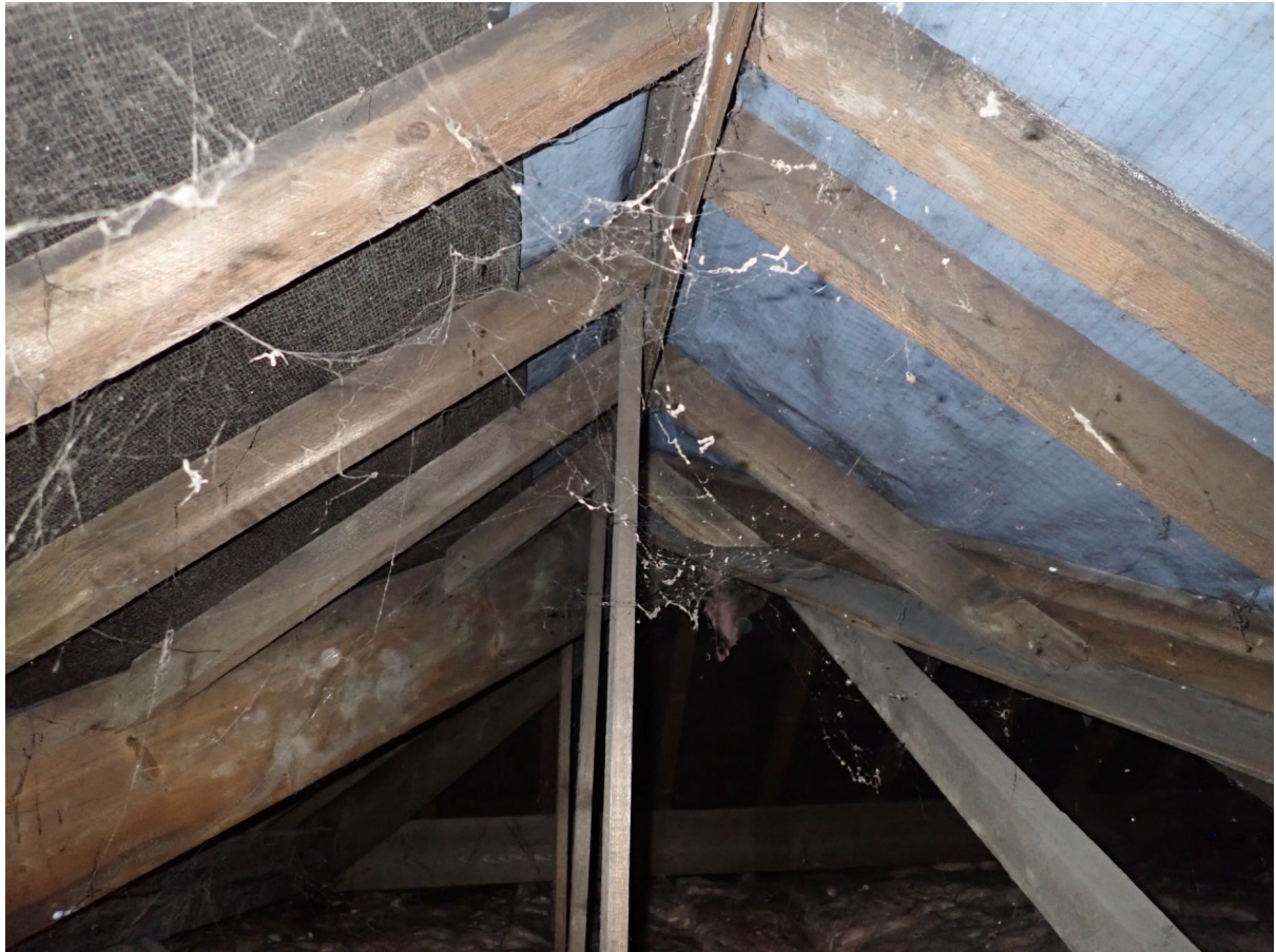
9 – Roof timbers are covered in dusty cobwebs.
