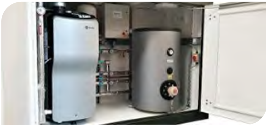
Figure 5. typical external packaged ASHP plant room
