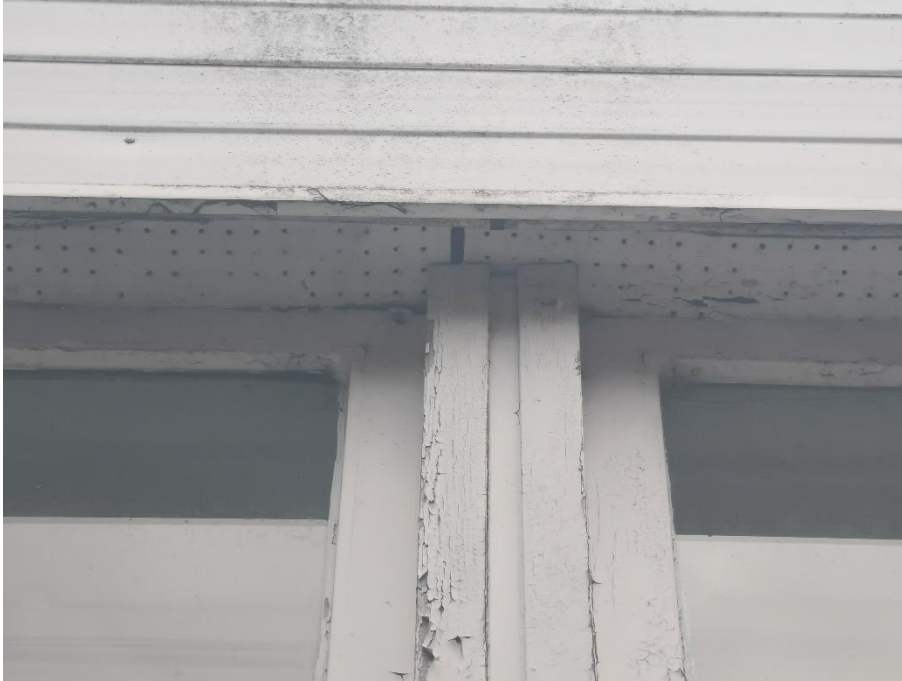
Photograph 5- Further gap on western elevation
