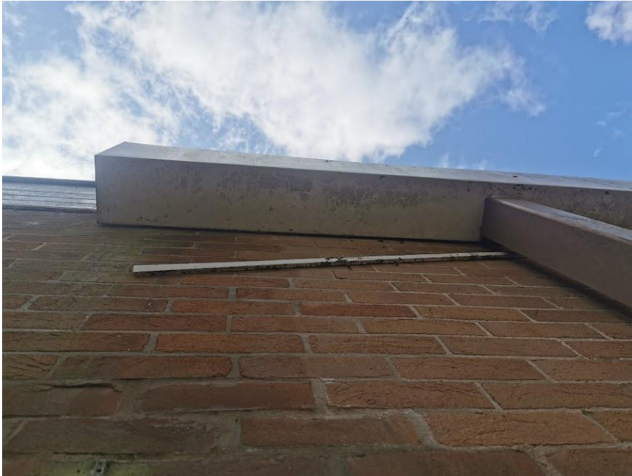
Photograph 7- Guttering gap on northern elevation
