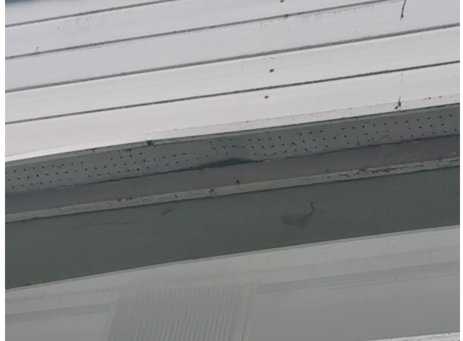
Photograph 4- Gap in western elevation
