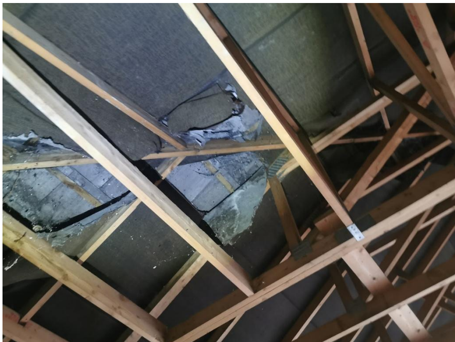
Photograph 11- Interior of B2, roofing felt gaps with cobwebbing
