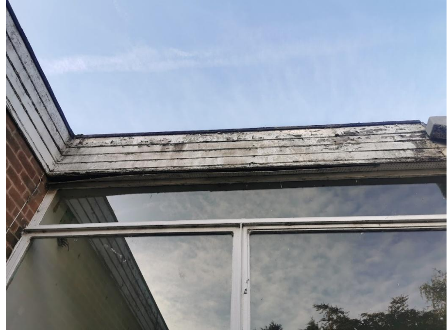
Photograph 10- Soffit gap in courtyard
