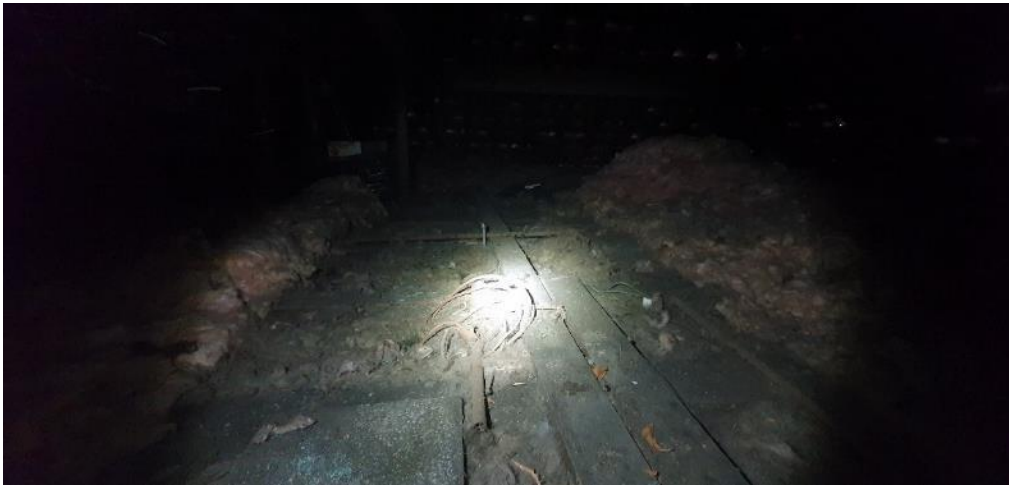
B1 – boarding around the loft hatch (pictured above).
