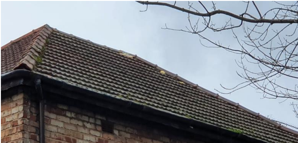
B1 – eastern elevation roof showing areas of expanding foam (pictured above).
