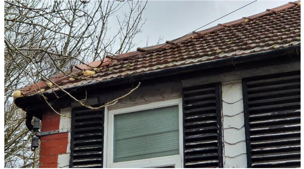
B1 – north western elevation roof showing areas of expanding foam (pictured above).
