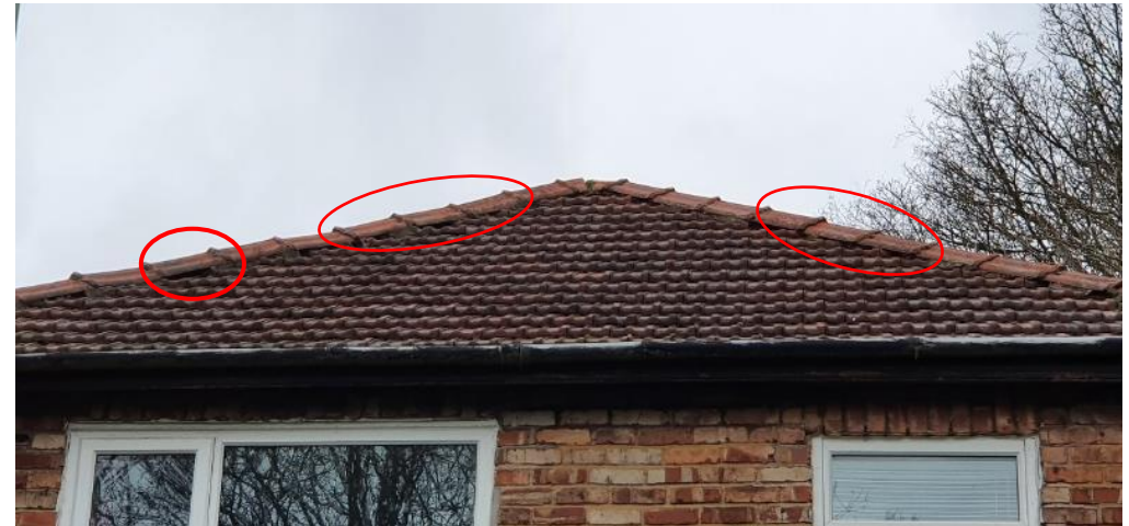
B1 – south eastern elevation roof showing areas of missing mortar (pictured above).
