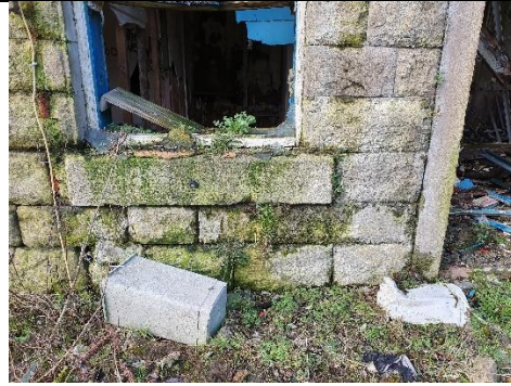
B3 Visible gaps within stonework 2020
