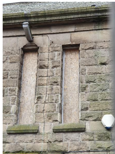
B1 Visible gaps beneath stone window ledge in 2020
