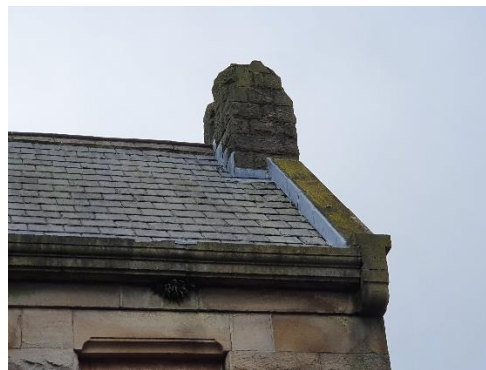
B1 Visible gaps within the ridge line and surrounding flashing in 2020
