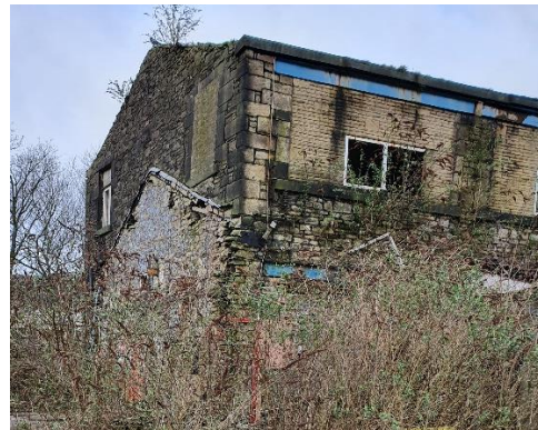
B2, demolished section to the southern elevation in 2020
