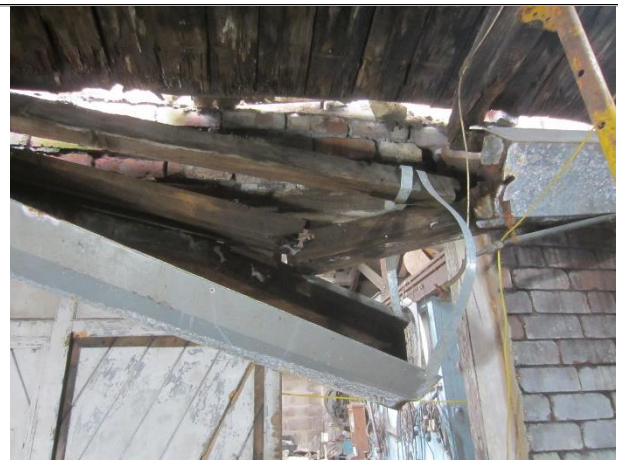
Photo 14: Interior of lean-to showing roof damage
