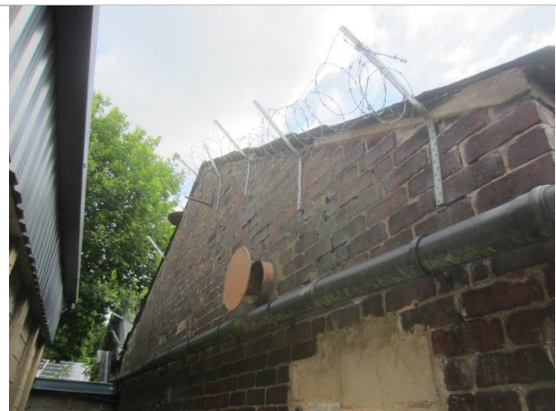
Photo 6: Barbed wire at western gable end of workshop
