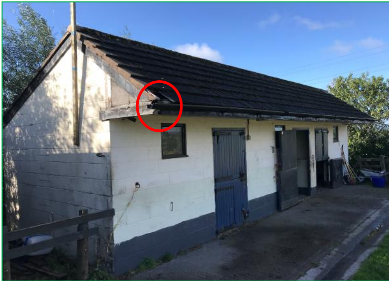
The stable building: Showing the one large gap in the roof at the northeast corner
