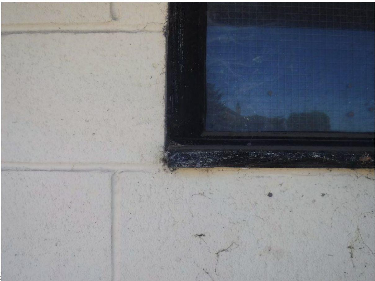
6 – Window and door frames are sealed into the walls with no suitable gaps.
