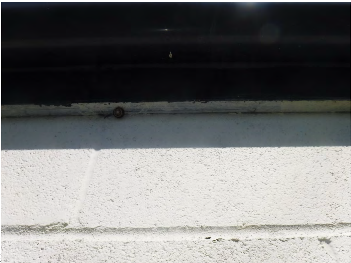
4 – Wooden fascia boards are fixed tightly against blockwork with no suitable gaps.
