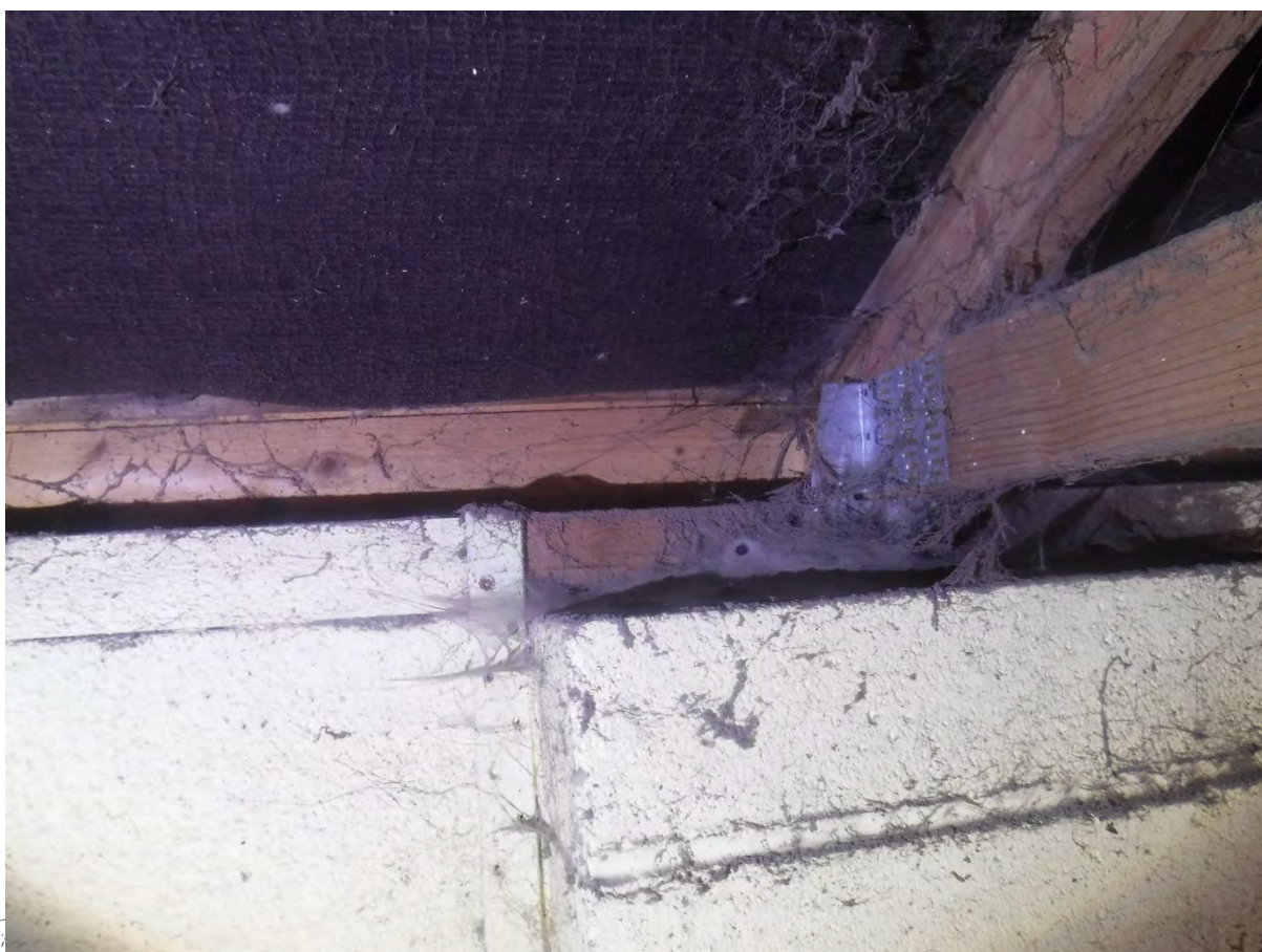
8 – Timbers are covered in dusty cobwebs with no gaps between timbers and blockwork.
