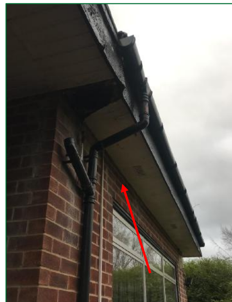
Showing the gap under the soffit on the southwest elevation
