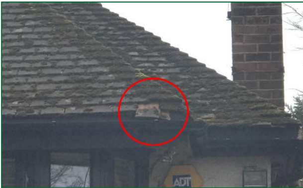
Showing slipped tiles on the northwest elevation
