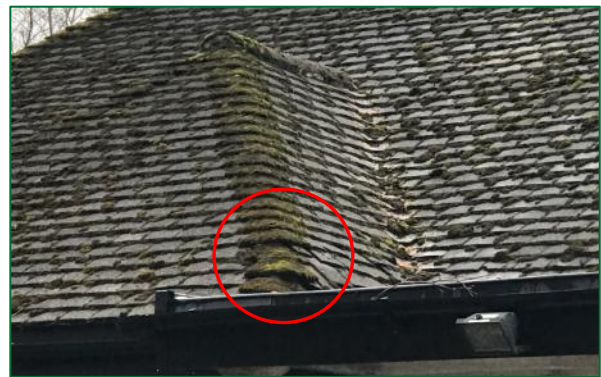
Showing lifted tiles on the northwest elevation
