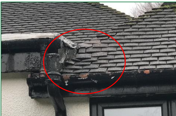
Showing lifted tiles on the northwest elevation
