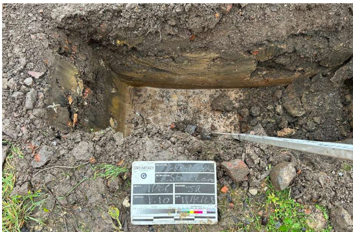
Photograph 24 – TP06 indicates basement is not continuous with the nearby wellton the south west.
