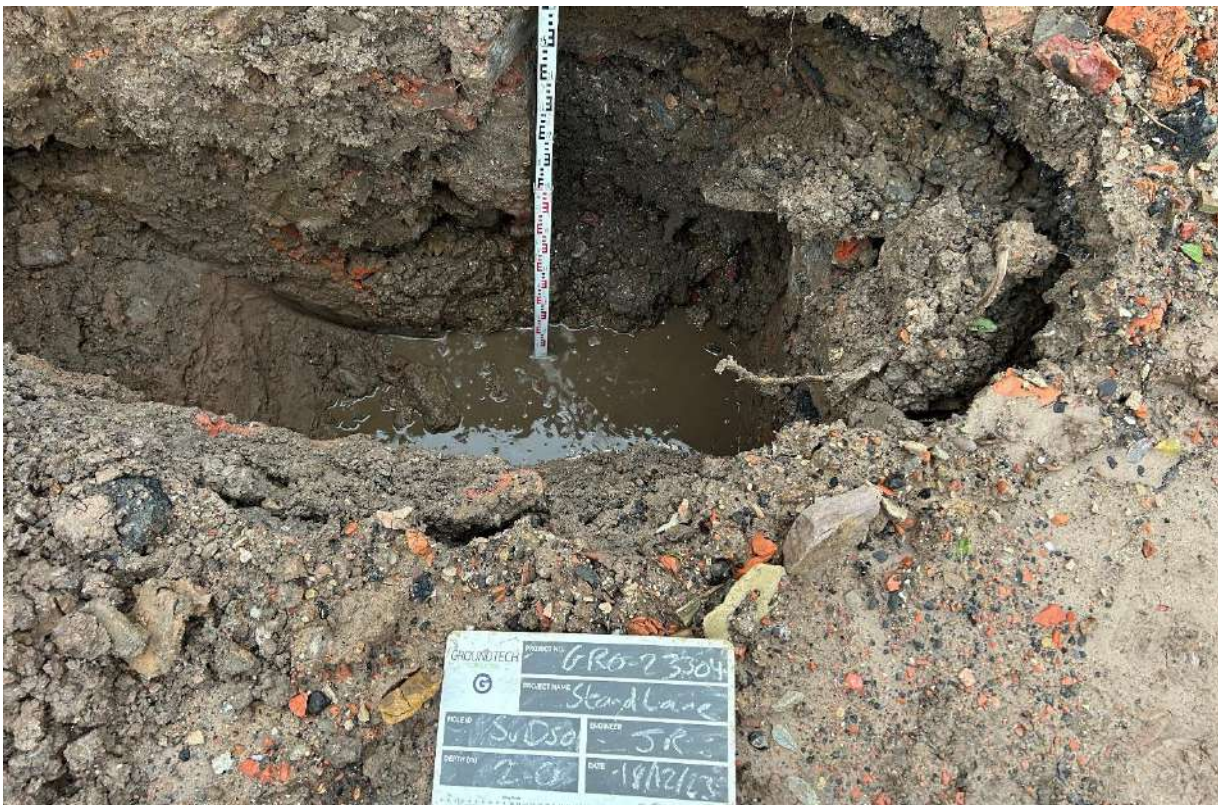
Photograph 18 – SuDS01 showing basement wall and perched water ingress.
