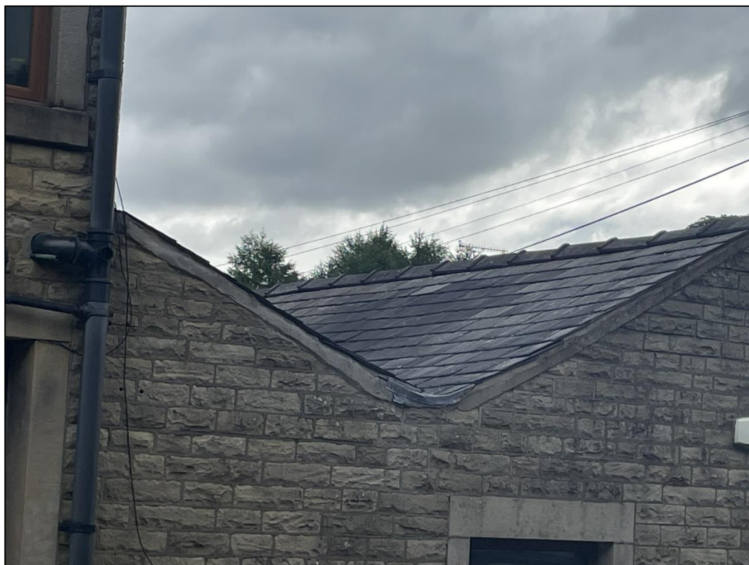
Plate 15 – Generally well-sealed slates on western roof pitch with minor gaps beneath ridge tiles.
