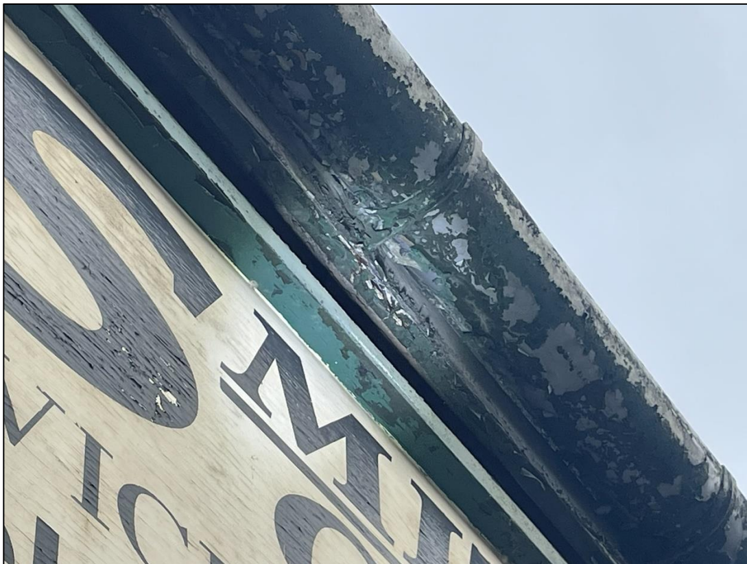
Plate 11 – PRF behind barge board on eastern elevation.
