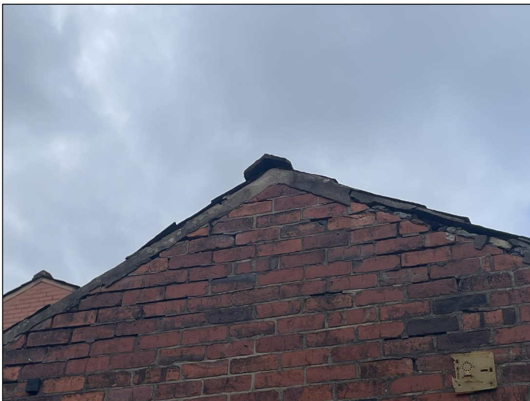
Plate 10 – Crevice opportunities beneath slates and at apex ridge tile where mortar has degraded on eastern gable verge.
