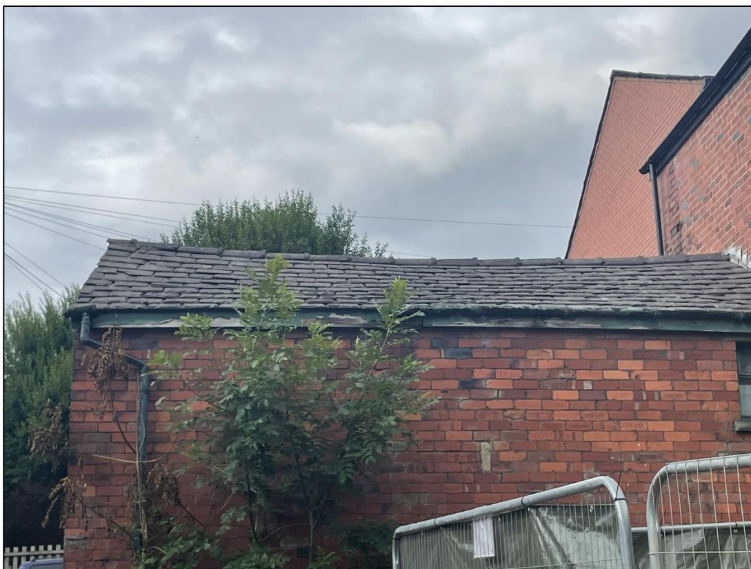
Plate 8 – Slipped slates on northern elevation.
