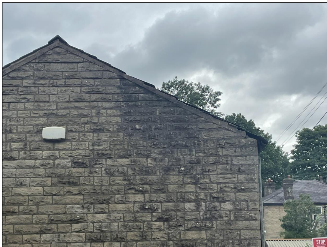
Plate 14 – PRFs on southern elevation where mortar is damaged presenting crevice opportunities beneath slates and ridge tiles.
