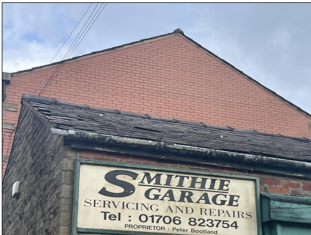
Plate 13 – Example of slipped slates on eastern elevation and gaps beneath ridge tiles.
