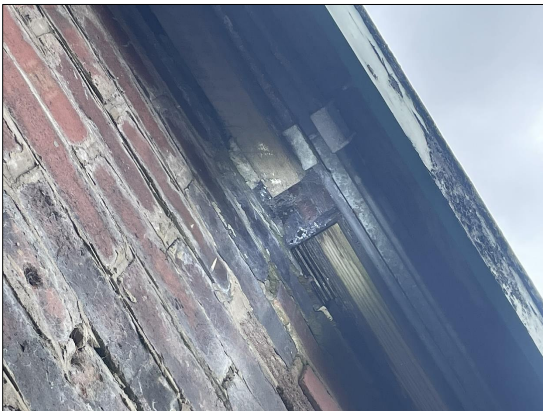
Plate 12 – Gap behind metal rolling shutter although cobwebbed on eastern elevation.
