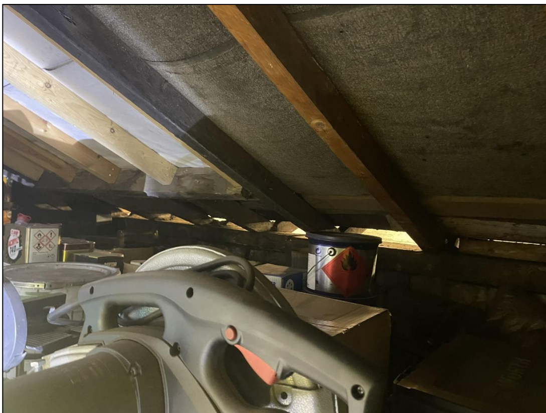
Plate 7 – Gaps at the base of the loft space.
