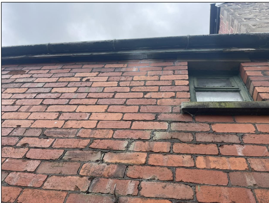
Plate 9 – Gaps behind barge board on northern elevation presenting internal access and to the wall plate.
