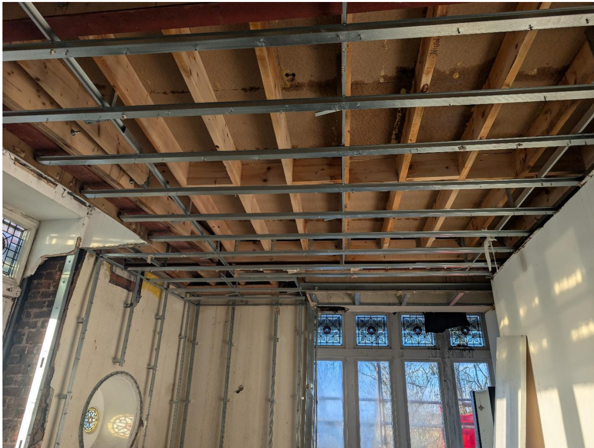
Picture 13 Soffit of 4th Floor In Front Section
