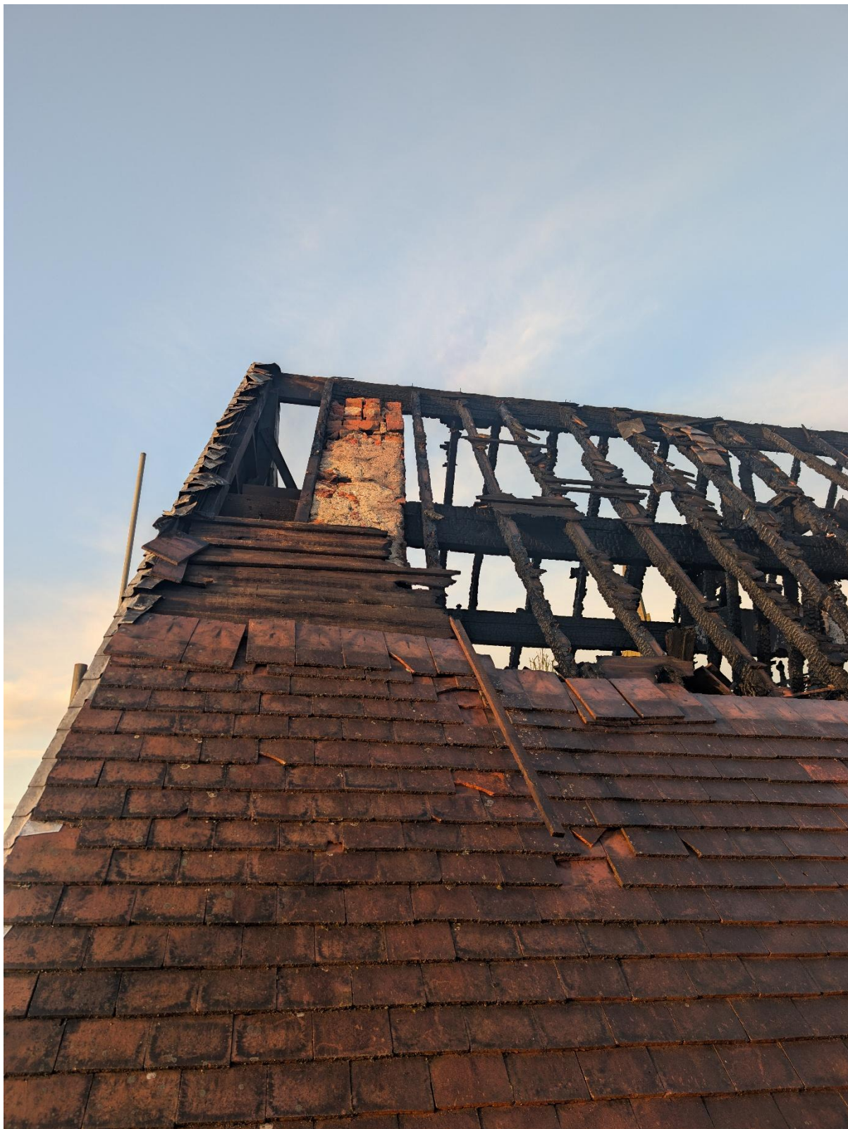
Picture 5 View on Front Gable - Slight Inwards Lean at Peak – Localised Outwards Displacement of Roof Overhang
