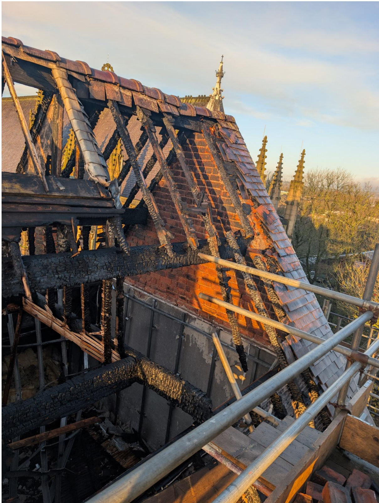
Picture 9 View on Rear Gable - Restraint from 4th Floor Lost
