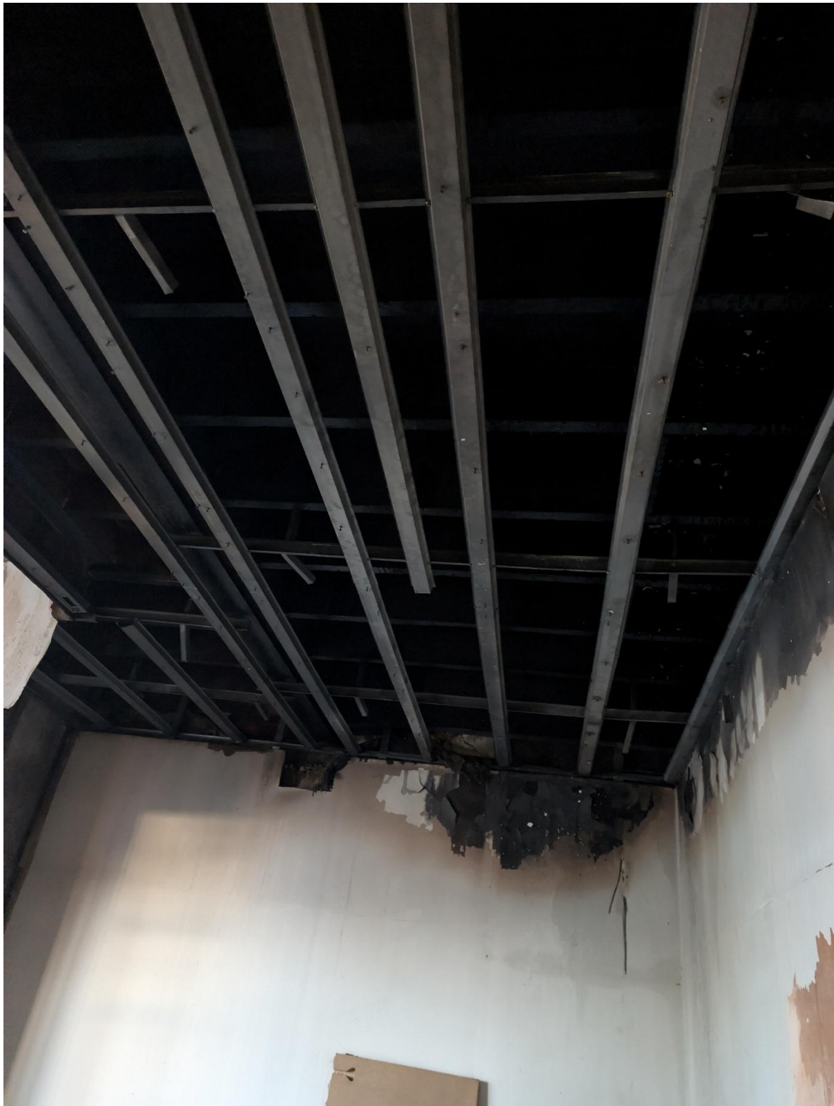
Picture 18 Soffit of 4th Floor Rear Left Section
