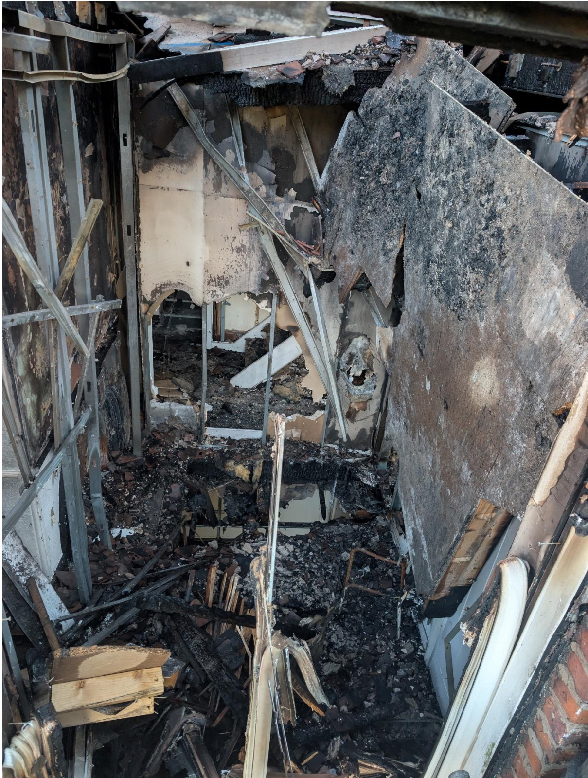
Picture 11 View Into 3rd Floor - 4th Floor Collapsed
