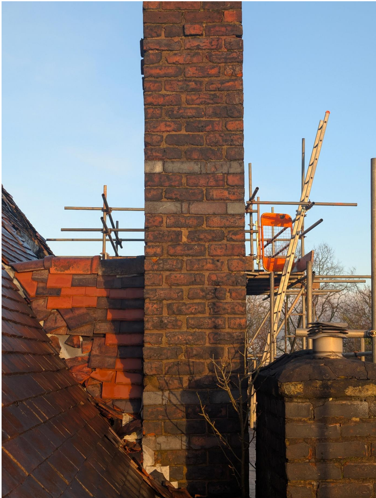
Picture 6 View on Front Left Chimney Stack - Slight Inwards Lean
