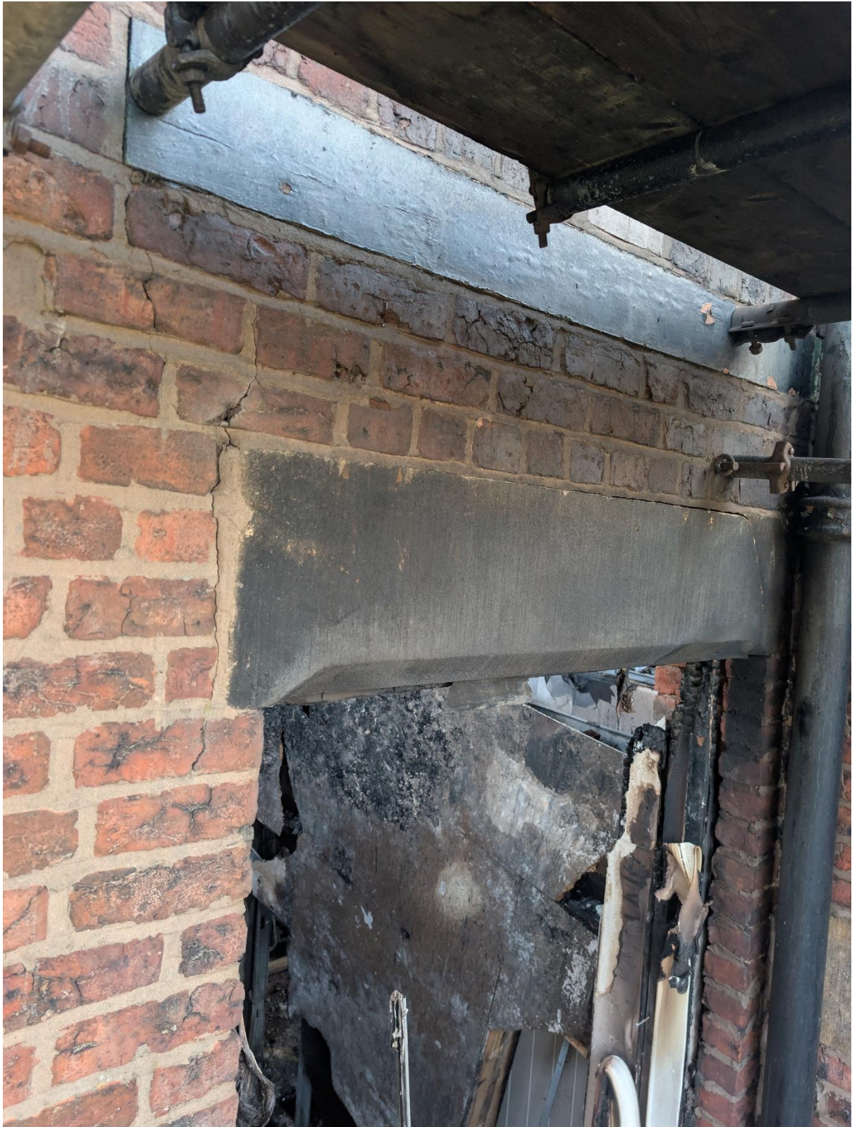
Picture 10 Fractured Lintel On Rear Elevation at 3rd Floor
