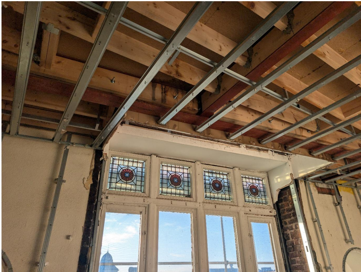
Picture 14 Soffit of 4th Floor In Front Section
