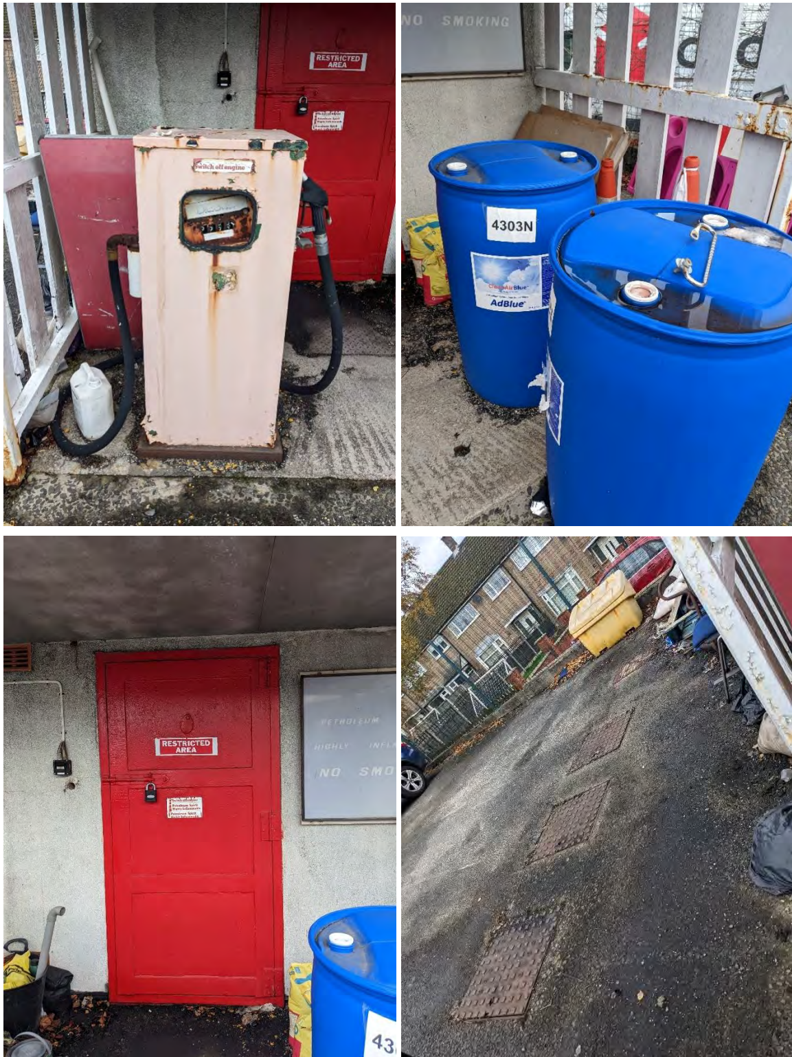
Figure 4: Photographs of the diesel pump, AdBlue, petroleum spirit storage and interceptor
