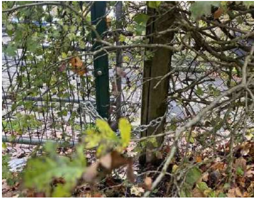
Photo 13 - Unsecured gap between legacy chain-link fencing and newer mesh fencing to the roadside boundary, resulting in a breach of the secure line and enabling unauthorised access on the south boundary
