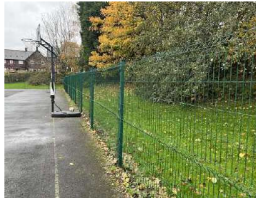
Photo 4 - 1.8m perimeter fencing that does not meet DfE minimum height requirements for safeguarding boundaries.
