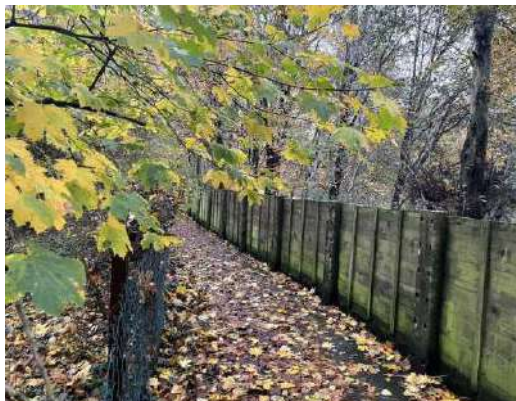
Photo 11 - Public footpath directly adjoining the school perimeter, where low and deteriorated chain-link fencing provides inadequate separation between members of the public and the school grounds.
