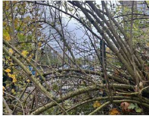
Photo 14 - 1.8m perimeter fencing that does not meet DfE minimum height requirements for safeguarding boundaries
