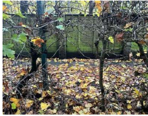
Photo 8 - Complete collapse of boundary fencing allowing unrestricted access to a public footpath adjacent to a motorway, representing an extreme safeguarding risk.
