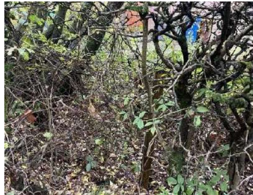
Photo 2 - Full opening in perimeter fencing to the south-west boundary, creating unrestricted public access and a critical safeguarding risk
