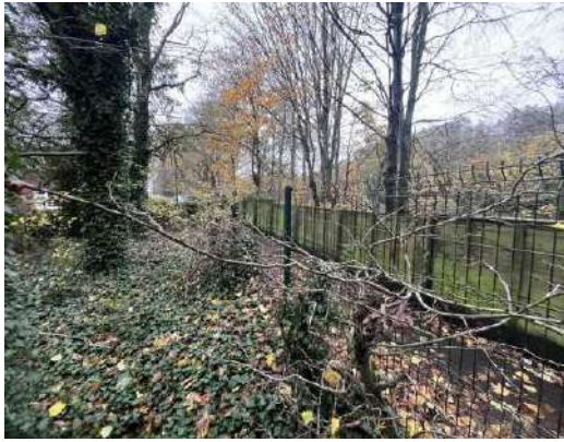
Photo 7 - 1.8m perimeter fencing that does not meet DfE minimum height requirements for safeguarding boundaries.
