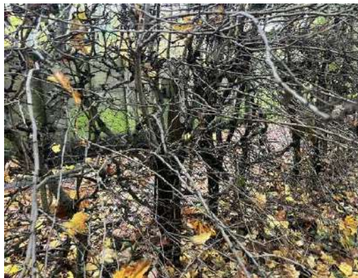
Photo 9 - Low level chain link fencing Low-level, life-expired chain-link boundary fencing providing ineffective safeguarding and unrestricted access to the school site
