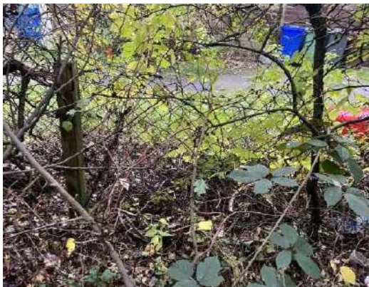
Photo 3 - Low level chain link fencing Low-level, life-expired chain-link boundary fencing providing ineffective safeguarding and unrestricted access to the school site
