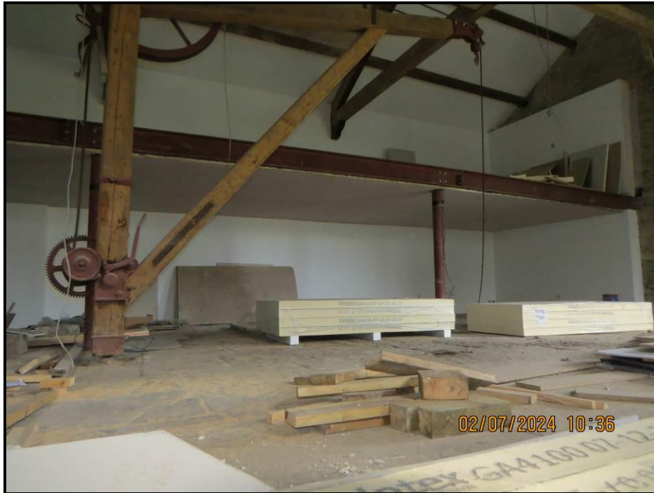
030 Crane and loading platform
