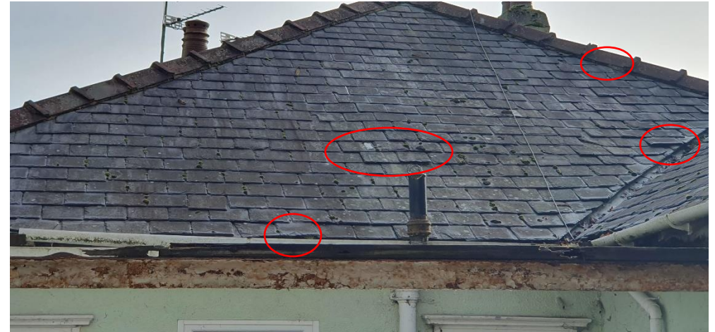
B1 – western elevation roof with highlighted lifted tiles and gaps
