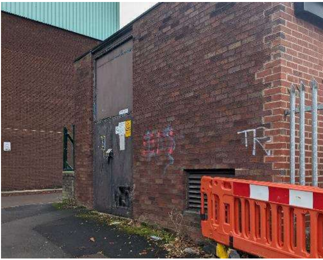
Figure 13 – An electricity sub-station adjacent to the northeastern site boundary, looking southeast.
