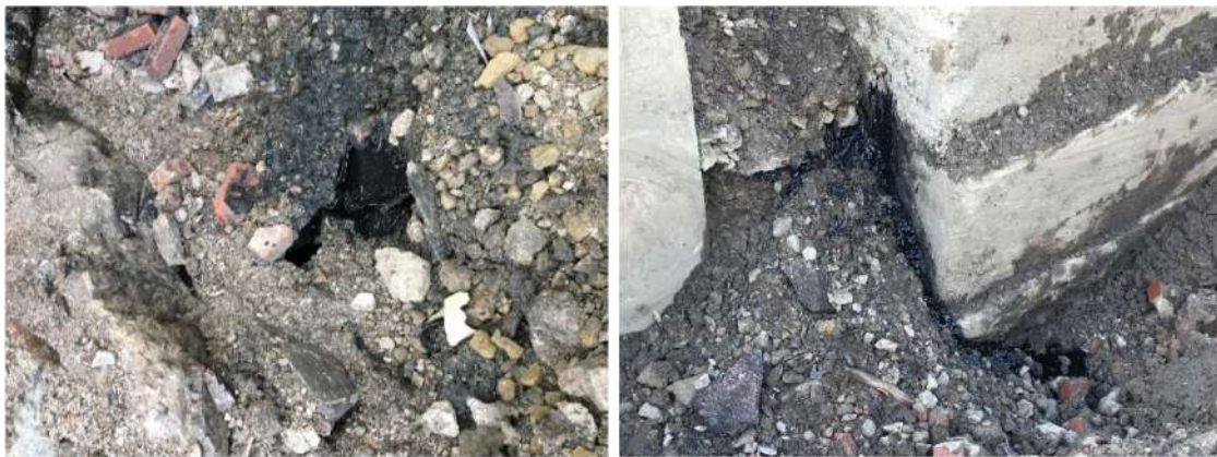
Figure 5 - E3P photos showing 'hydrocarbon liquid' down gradient of USTs.
