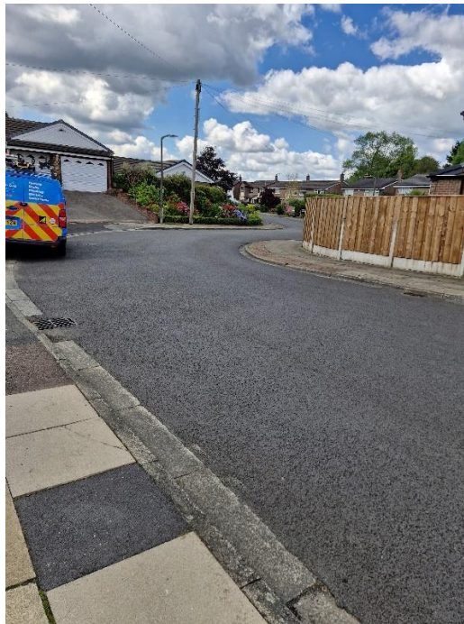
planting obstructing visibility
