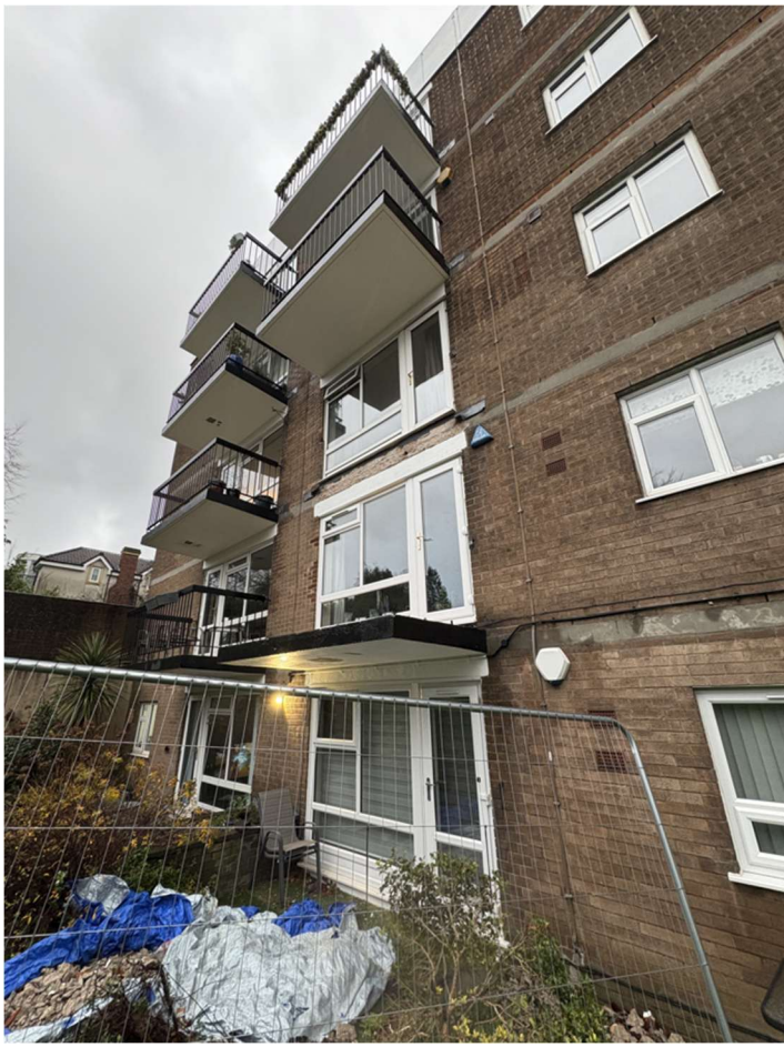
Photo of collapsed balcony
