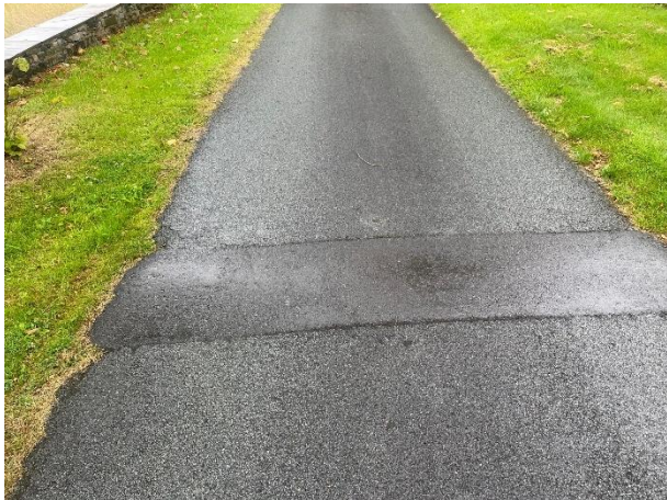
9. Access Rd 25m from Turton Rd, showing previous repair
