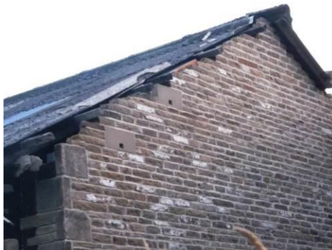
Example of Forticrete boxes in situ
