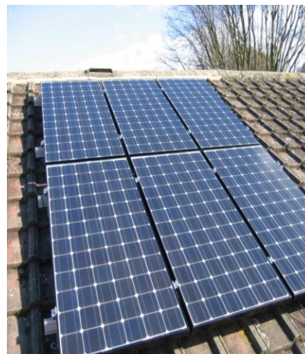
Figure 5 - Photovoltaic array on a pitched roof
