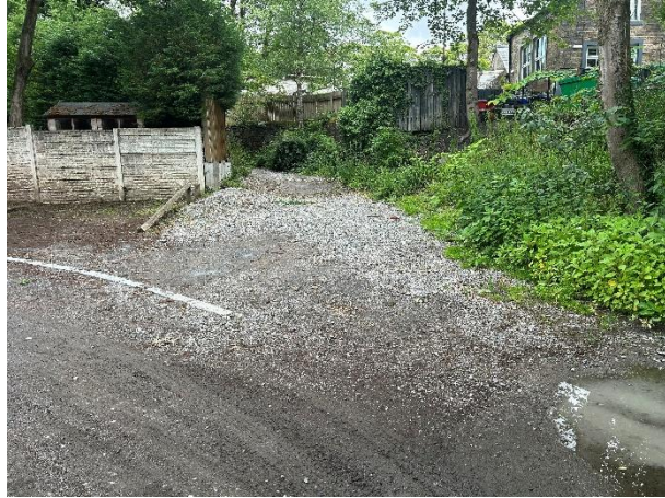
Bottom of bridleway showing stone surfacing washed down
