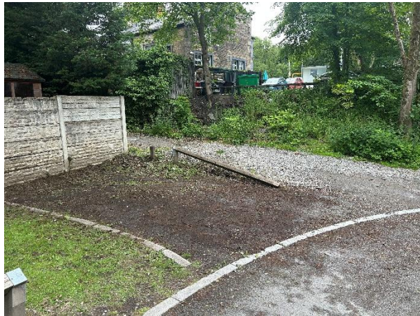
Damaged timber knee rail adj bridleway
