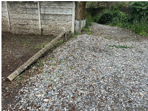
Damaged timber rail and washed stone
