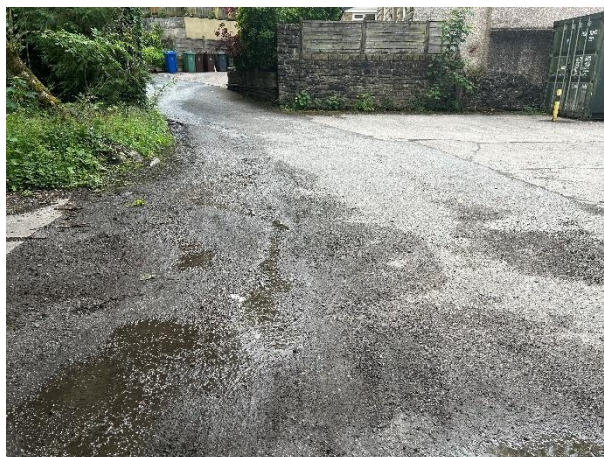
Poor surfacing and water run off outside Halter Inn
