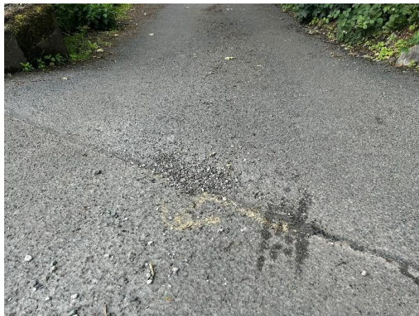
Boundary line at exit/entrance appears to be marked for patch reinstatements
