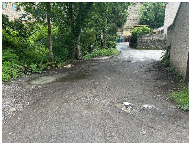
Poor road condition including puddles outside Halter Inn
