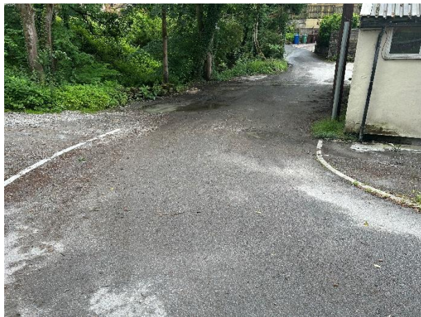
Road condition poor next to telegraph pole
