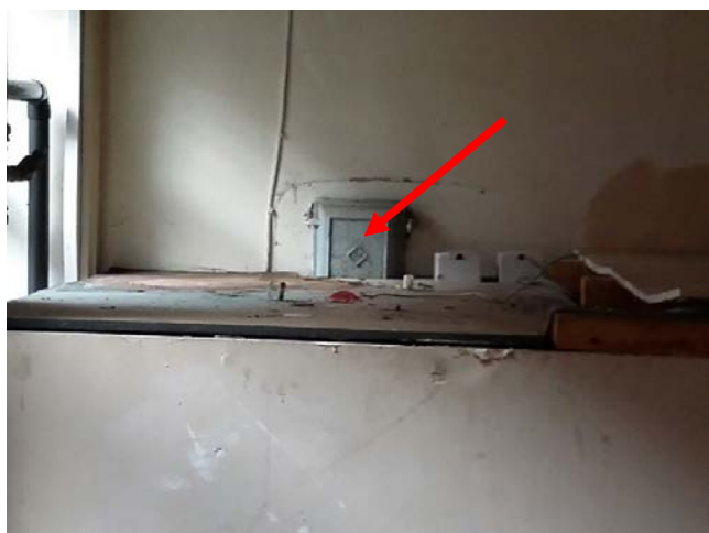
Sample No: No Sample G.09 Kitchen area Old fuse box above WC Flash guards containing: Chrysotile
