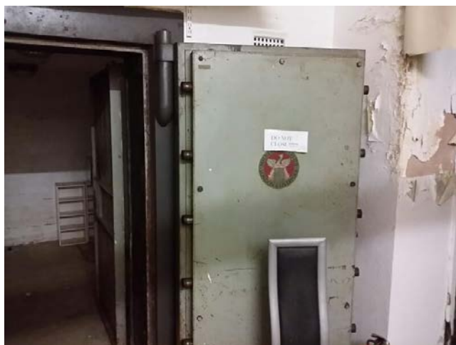
Safe door to B.09 (may have ACMs internally)
