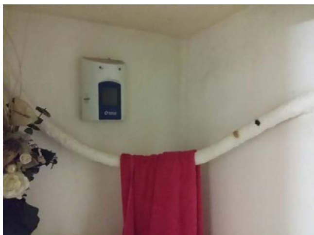
Sample No: 21/11/B/25/PK22 B.05 WC Electrical cable Woven wrap No Asbestos Detected
