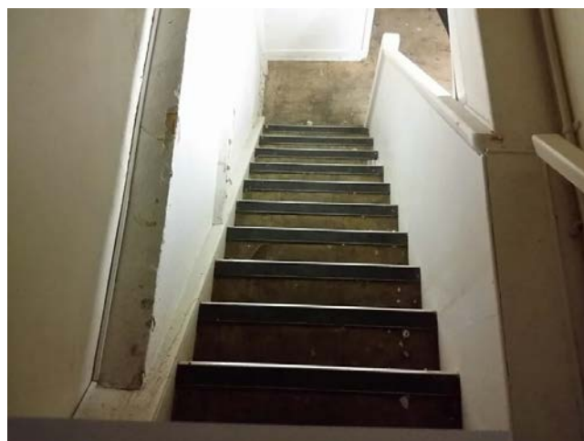
Sample No: 21/11/B/25/PK21 G.13 Stairwell Stairs Vinyl covering No Asbestos Detected
