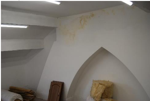
Damp from Chimney
