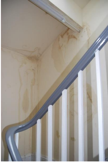
Dampness to stairwells
