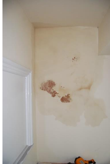
Damaged plaster to landing area
