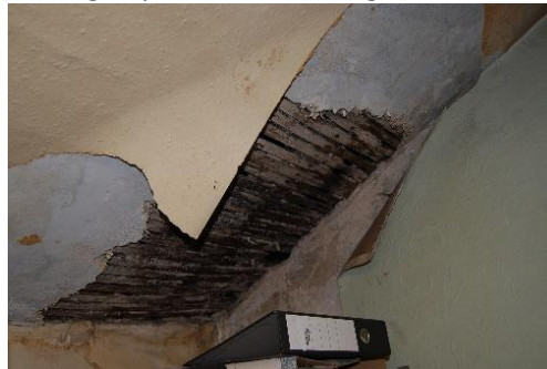
Dampness affecting ceilings
