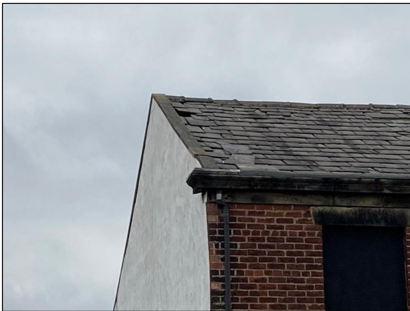
Photograph 11 showing the missing roof tile
