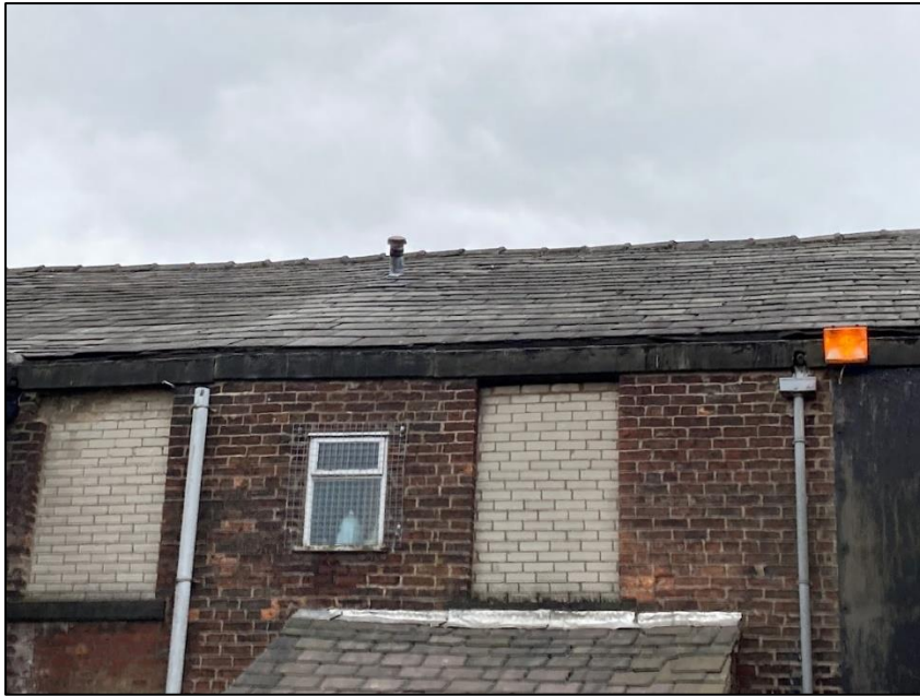
Photograph 10 showing a section of the roof
