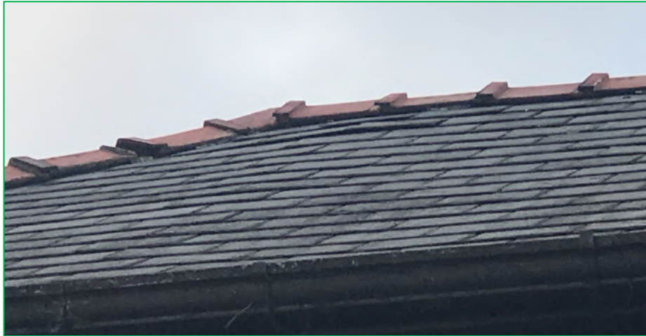
Showing crevices under lifted and slipped slates and under slipped ridge tiles
