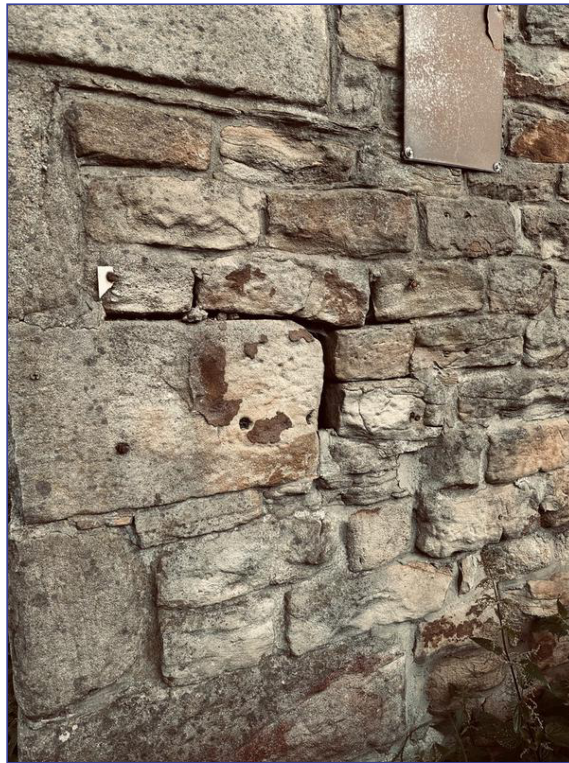
Photo 66 - Cracks to external stone work mortar need pointing
