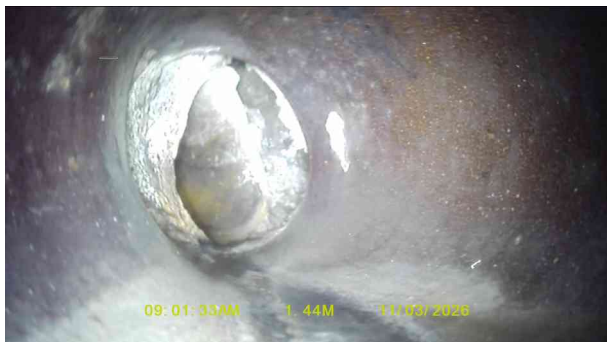
3, 00:00:11, 1.44 m Line deviates left
