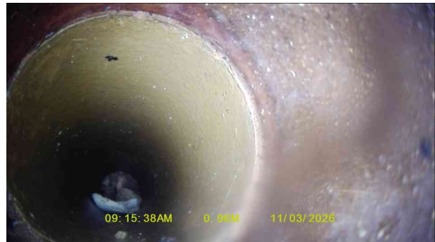
4, 00:00:18, 0.96 m Joint displaced, medium
