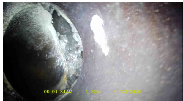
4, 00:00:12, 1.72 m Broken pipe at joint from 12 o'clock to 4 o'clock
