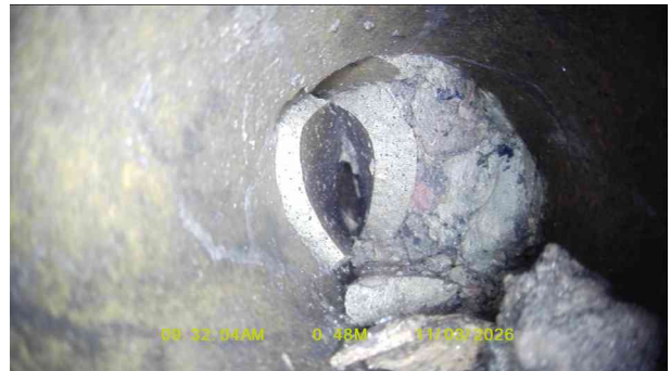
4, 00:00:19, 0.48 m Collapsed drain or sewer, 100% cross-sectional area loss
