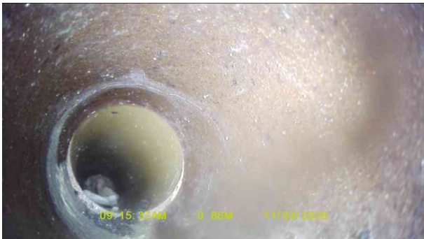
3, 00:00:17, 0.86 m Crack, circumferential from 6 o'clock to 2 o'clock
