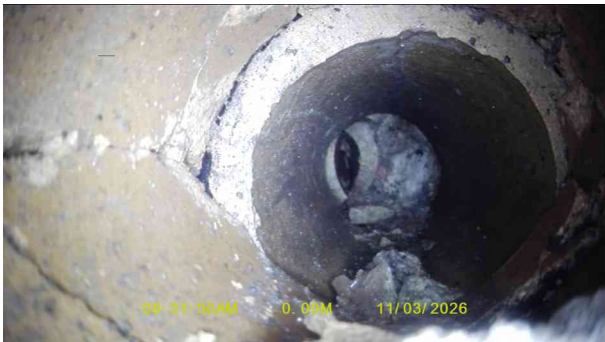
3, 00:00:12, 0.10 m Joint displaced, large
