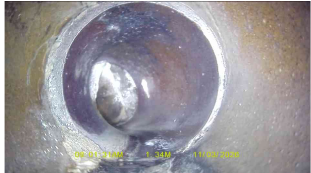
2, 00:00:09, 1.34 m Joint displaced, large
