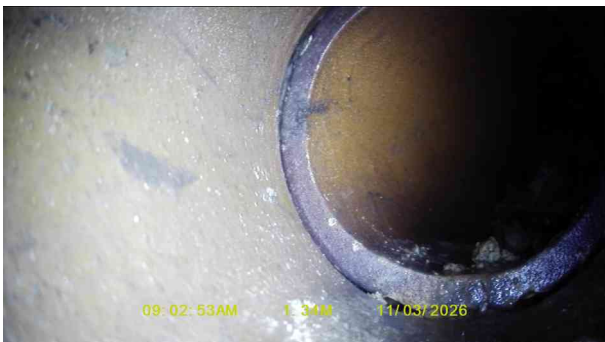
3, 00:00:22, 1.34 m Joint displaced, large
