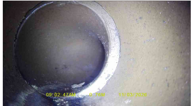
2, 00:00:16, 0.76 m Joint displaced, large
