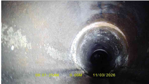
1, 00:00:04, 0.10 m Joint displaced, medium
