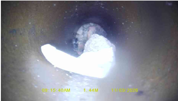
5, 00:00:20, 1.44 m Other obstacles, pipe material in invert at 6 o'clock, 45% cross-sectional area loss
