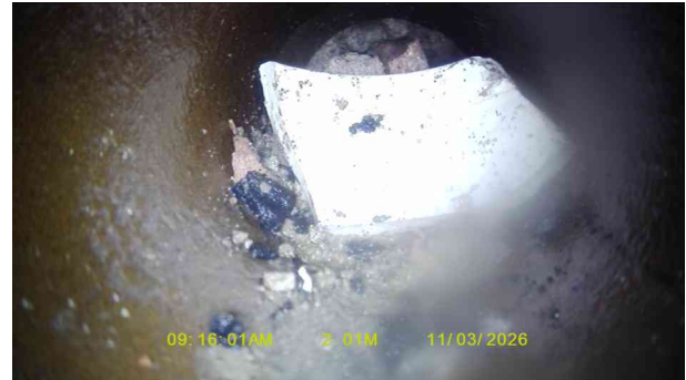
6, 00:00:41, 2.01 m Other obstacles, brick or masonry in invert from 12 o'clock to 12 o'clock, 100% cross-sectional area loss
