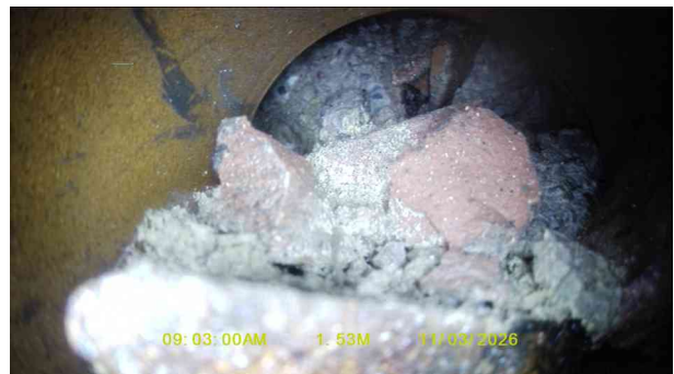
4, 00:00:28, 1.53 m Other obstacles, brick or masonry in invert from 12 o'clock to 12 o'clock, 100% cross-sectional area loss
