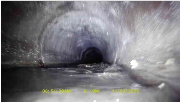
1, 00:00:11, 0.19 m Settled deposits, fine, 20% cross-sectional area loss, start
