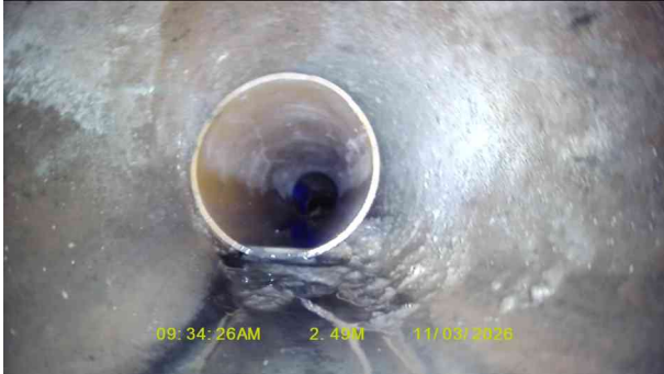
1, 00:00:16, 2.49 m Joint displaced, large
