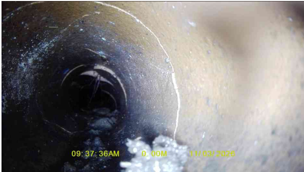
1, 00:00:04, 0.00 m Crack, circumferential from 8 o'clock to 4 o'clock
