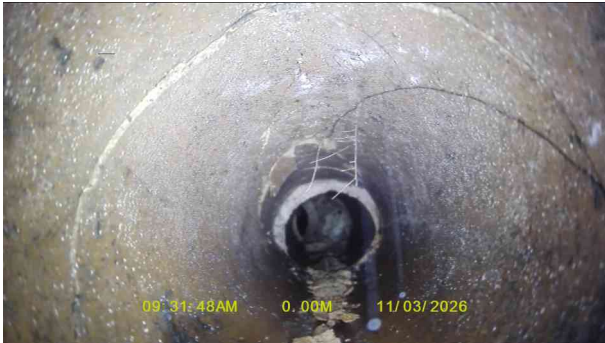
1, 00:00:03, 0.00 m Crack, circumferential from 8 o'clock to 4 o'clock
