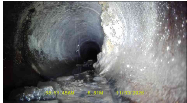
4, 00:00:37, 6.81 m Other obstacles, brick or masonry in invert at joint from 1 o'clock to 5 o'clock, 5% cross-sectional area loss
