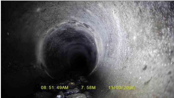
5, 00:00:40, 7.58 m Settled deposits, fine, 10% cross-sectional area loss, change
