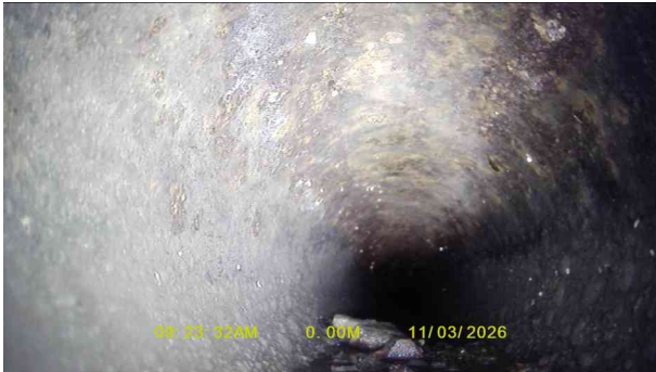
1, 00:00:03, 0.00 m Settled deposits, fine, 10% cross-sectional area loss, start
