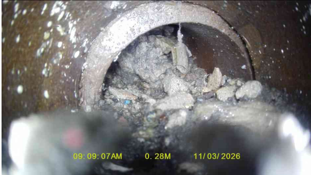
1, 00:00:10, 0.28 m Joint displaced, large
