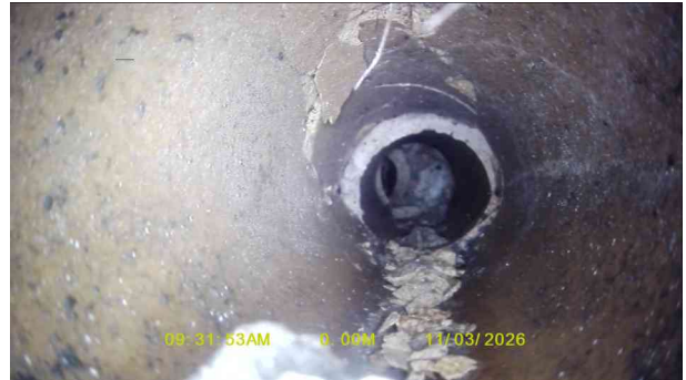
2, 00:00:09, 0.05 m Broken pipe at 11 o'clock
