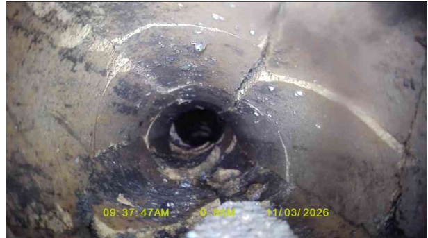
2, 00:00:14, 0.86 m Collapsed drain or sewer, 50% cross-sectional area loss
