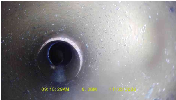
1, 00:00:08, 0.28 m Joint displaced, medium
