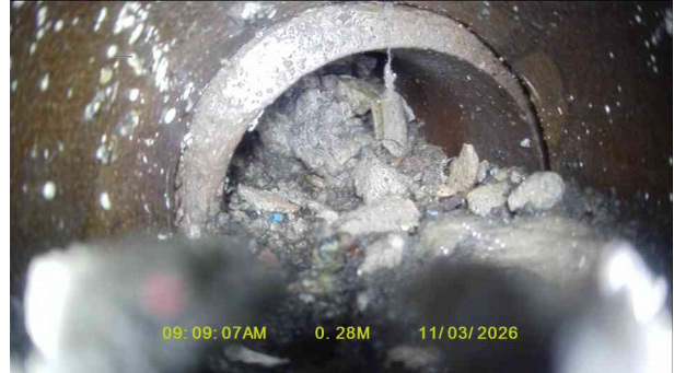
2, 00:00:10, 0.28 m Settled deposits, fine, 60% cross-sectional area loss
