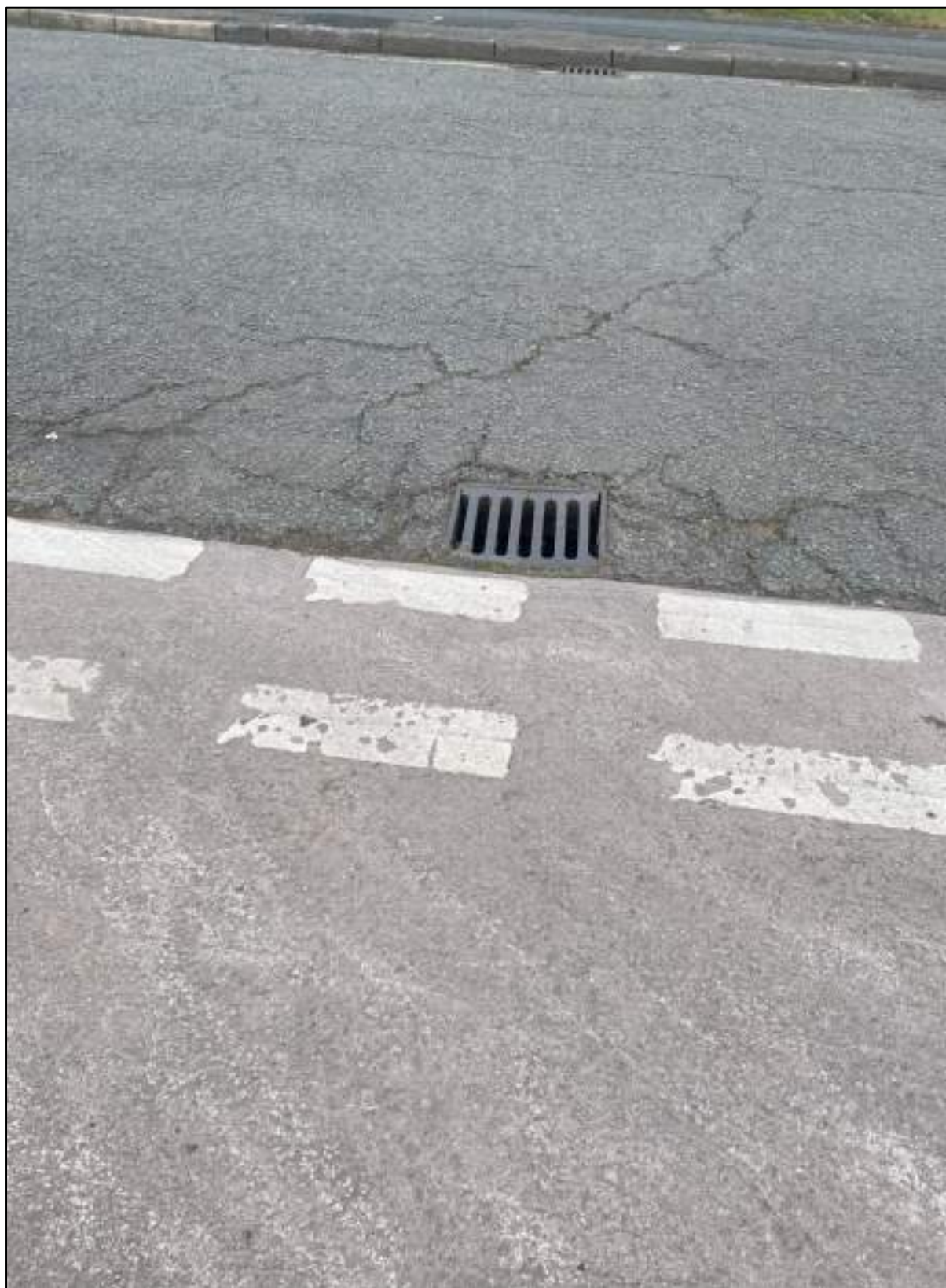
195m – Gulley at highway edge.
