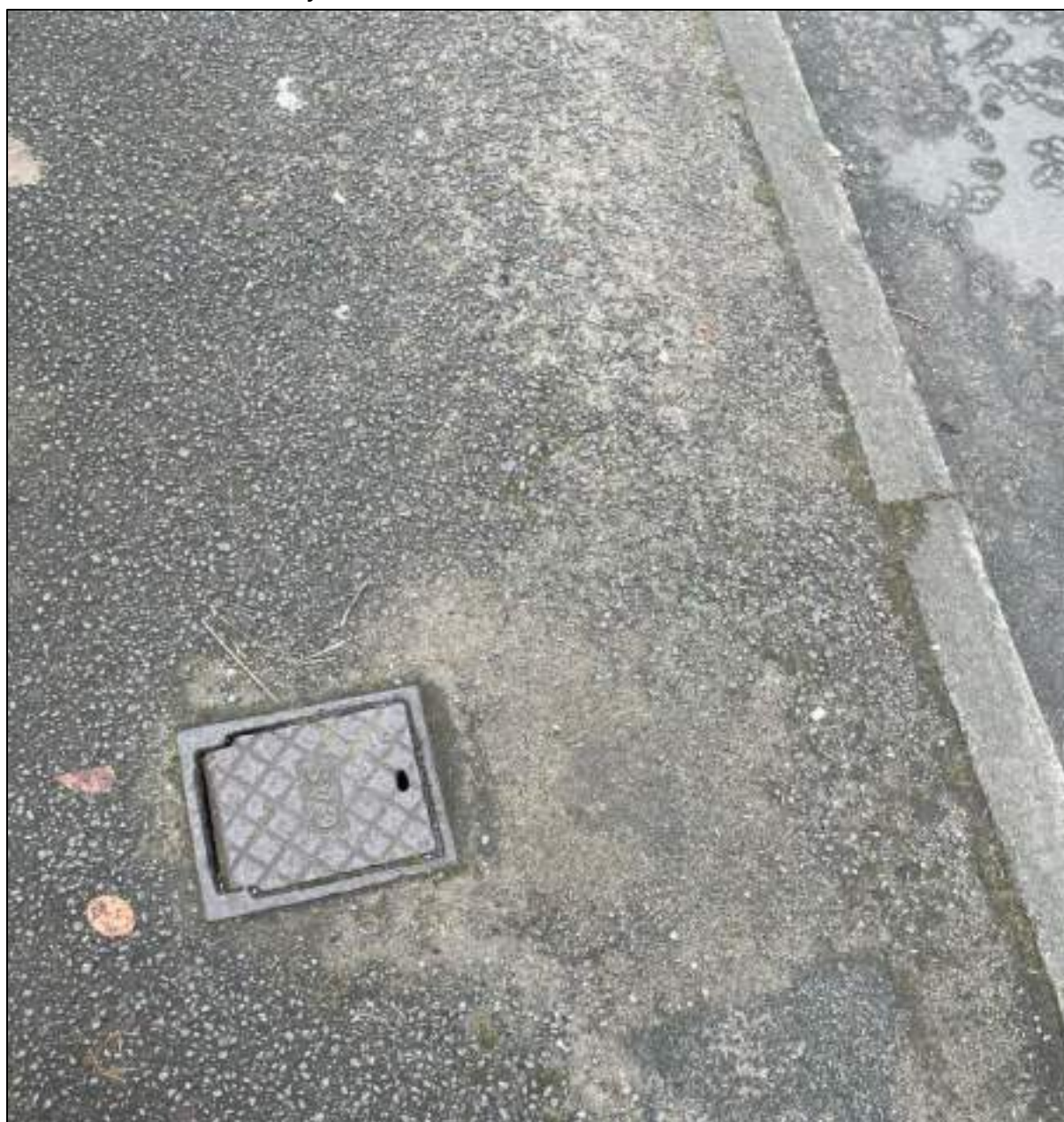
56m - Gas cover in footway.
