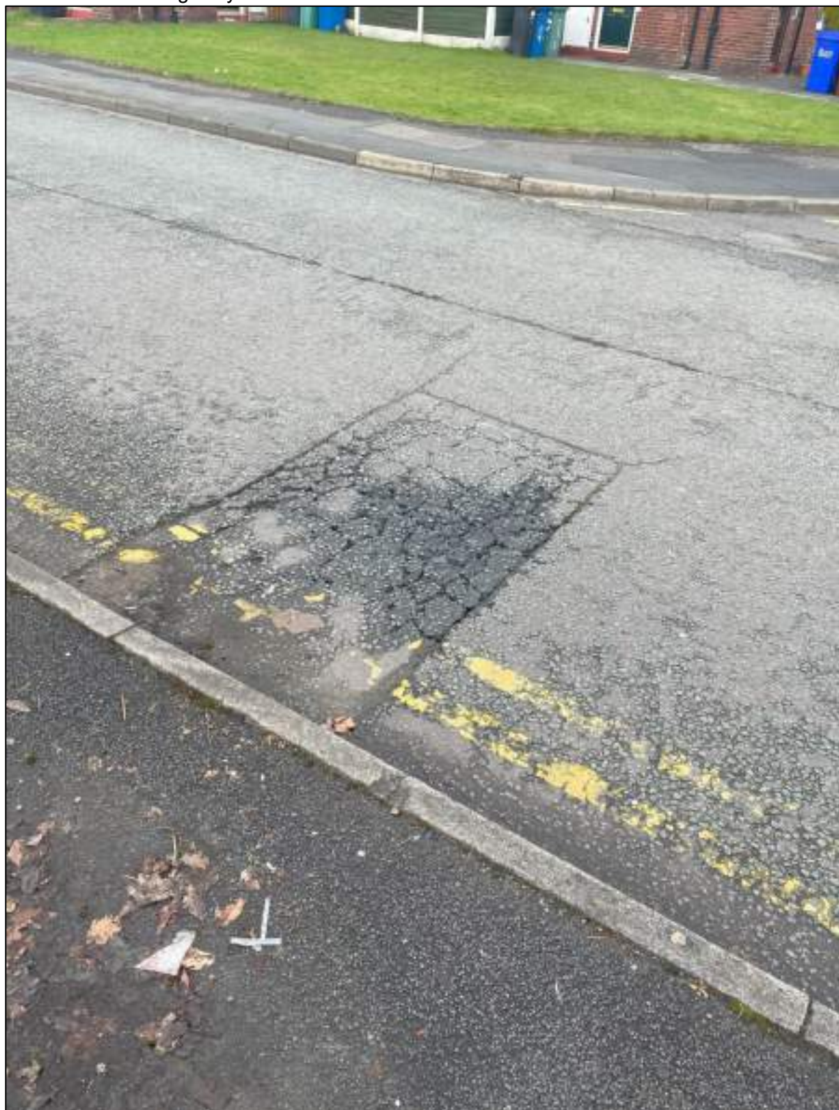
160m - Worn carriageway.
