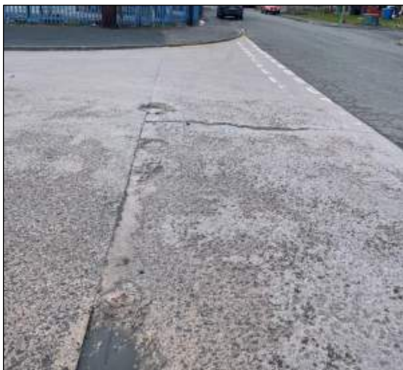
190m – Potholes in site access.
