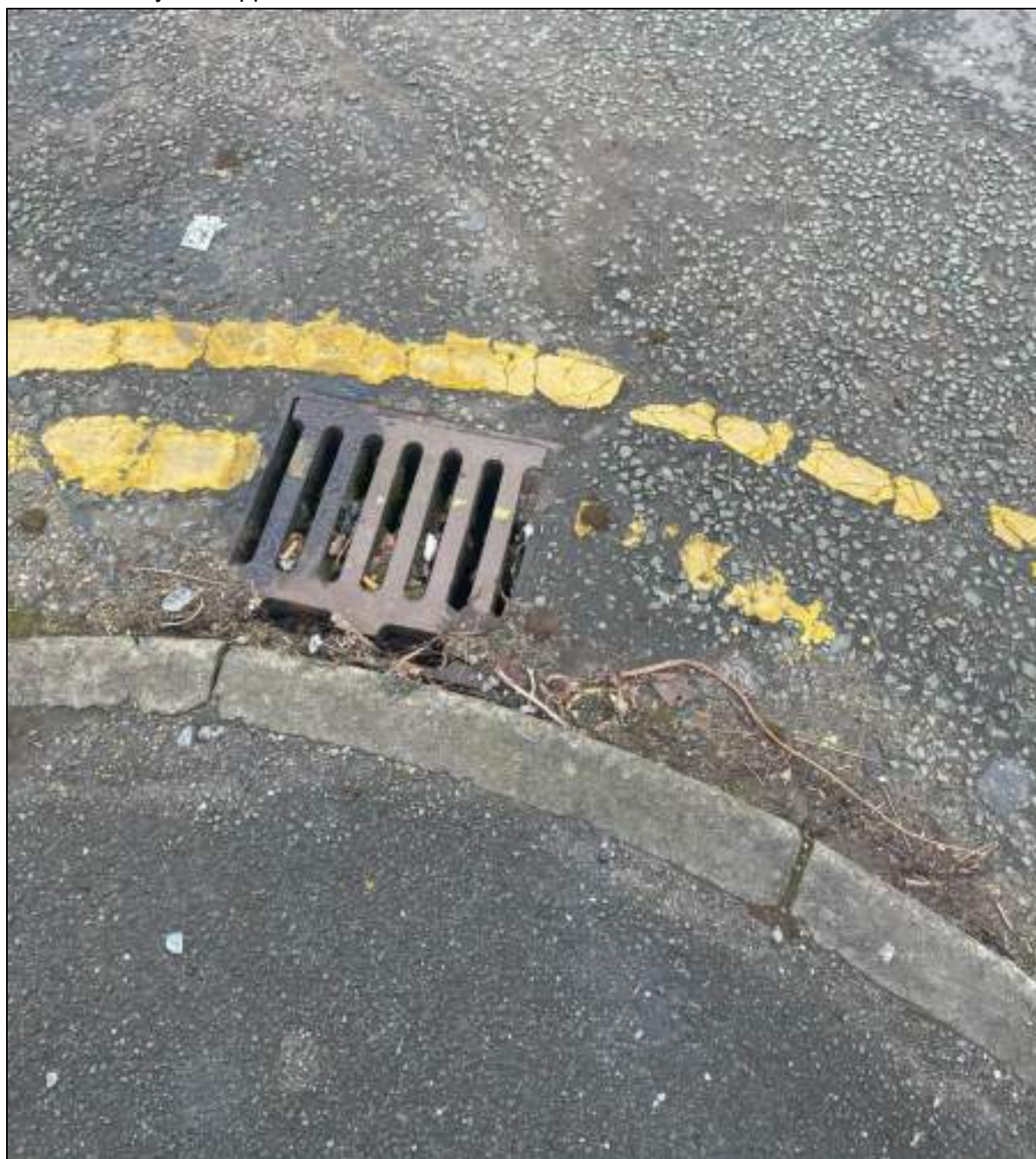
139m – Gulley at dropped kerb.
