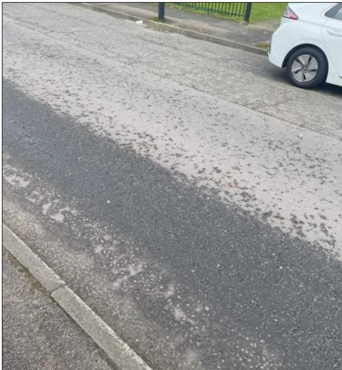
51m - Worn and cracked carriageway
