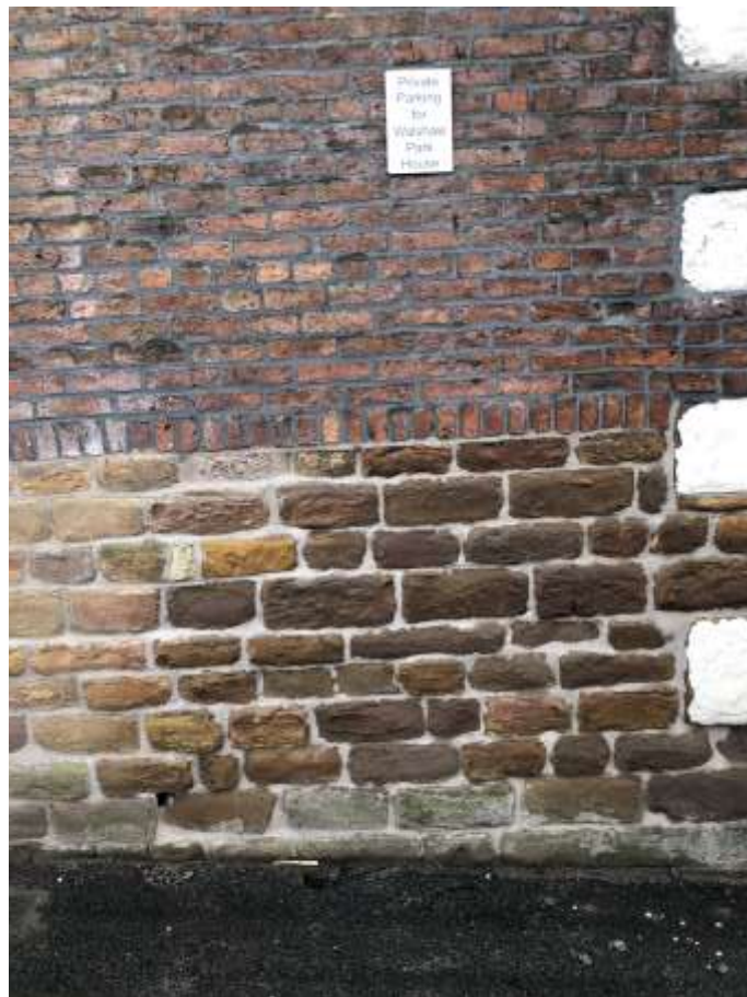
Image 8 – Car parking signage to side elevation
