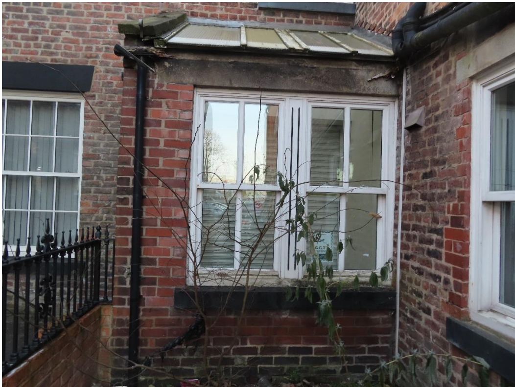
It can be seen by the reveal of this window that it has been created at a later period with a different type of brickwork and a more modern head and sill, therefore is not an original feature to the property, its heritage value there is limited.
