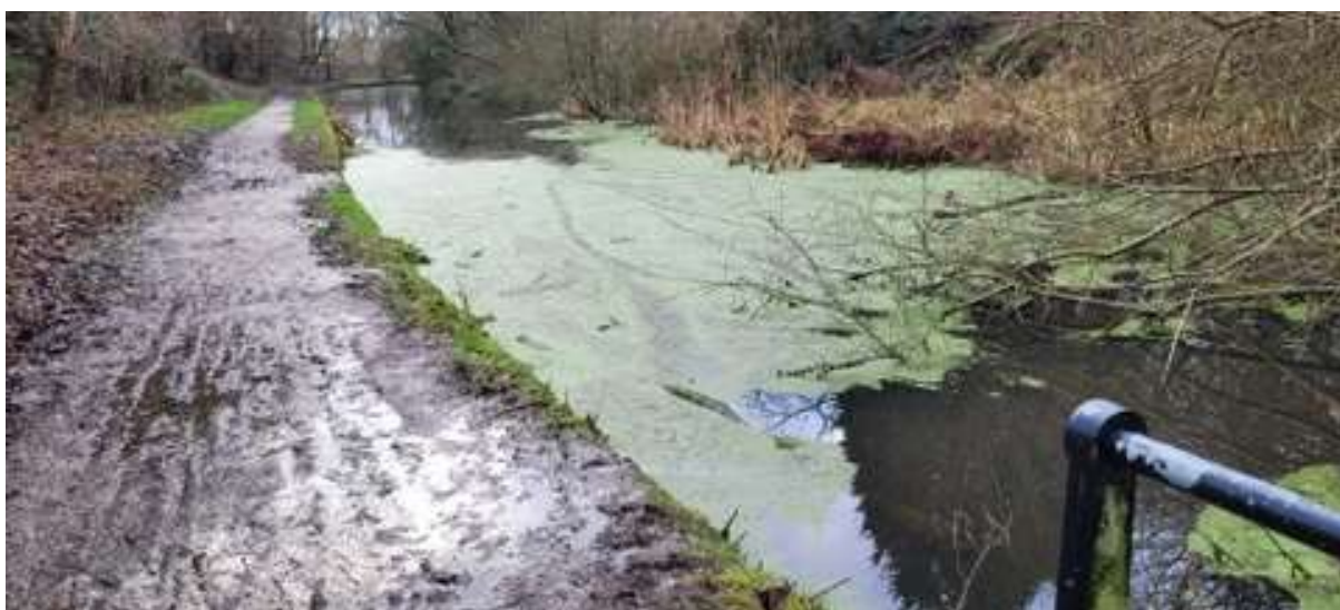
Photo 8 - Canal Bank adjacent to bridge and pipe, note bank lowered to this immediate areas
