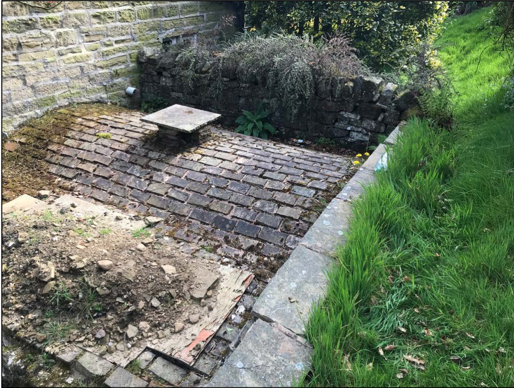
5.10 Modern stone setts to cellar roof. Defects including moss and vegetation growth, pointing loss.
