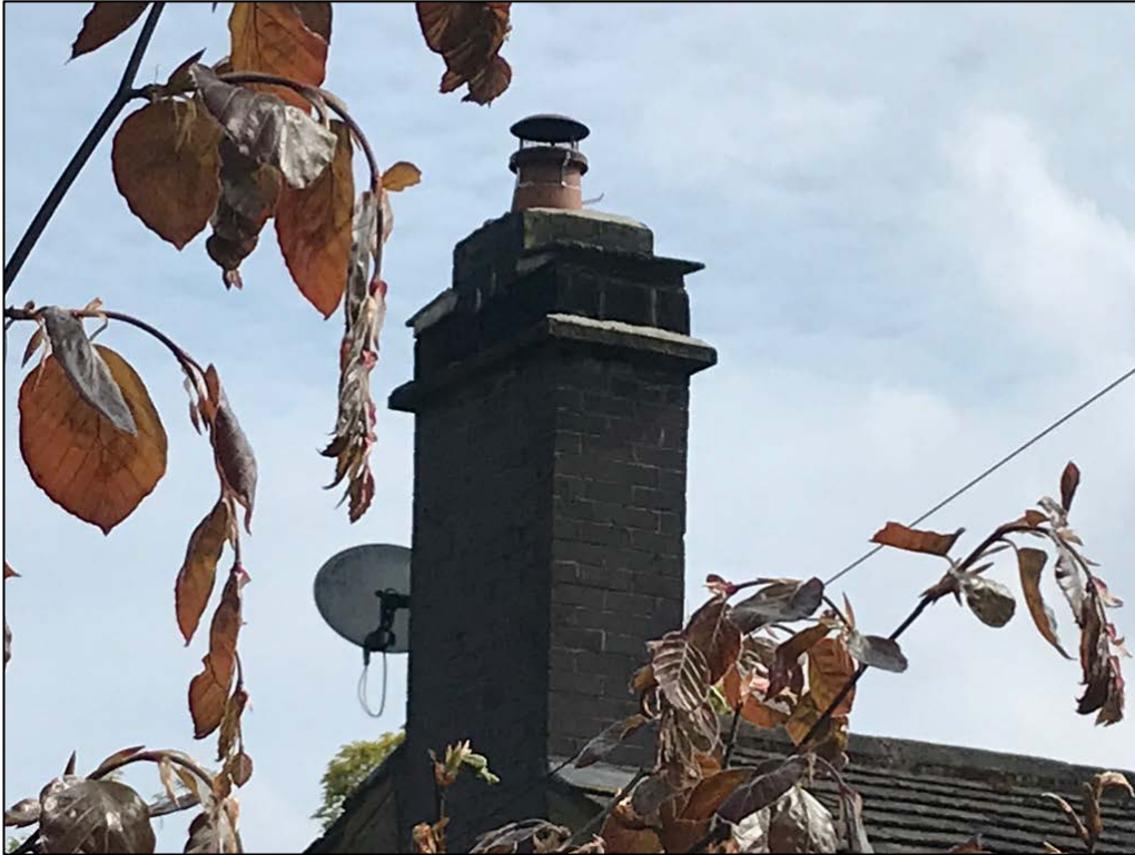
5.4 Incomplete mortar flaunching and moss growth to northern chimney stack.
