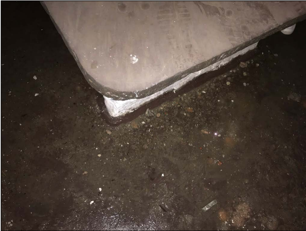
5.9 Significant water ingress to cellar area with standing water visible at ground level.
