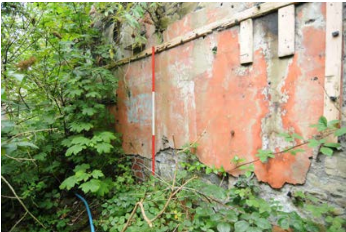
Photograph No : 36 Digital Ref: HOMI_HBR_0126 Direction: NW Description: Brick and stone beneath plaster in south gable of Building B
