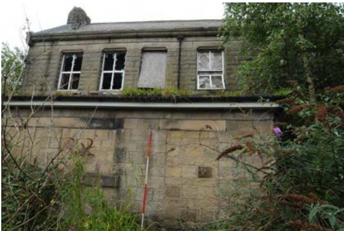
Photograph No : 17 Digital Ref: HOMI_HBR_0082 Direction: E Description: Blocked doorway in west elevation of single storey addition of Building A, first floor west elevation of Building A
