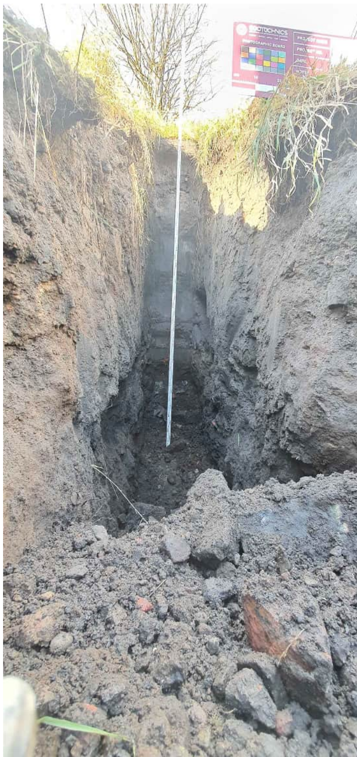
Trial Pit TPI02 (2)
