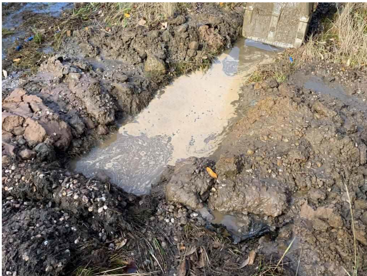
Trial Pit TPI 12 (2)
