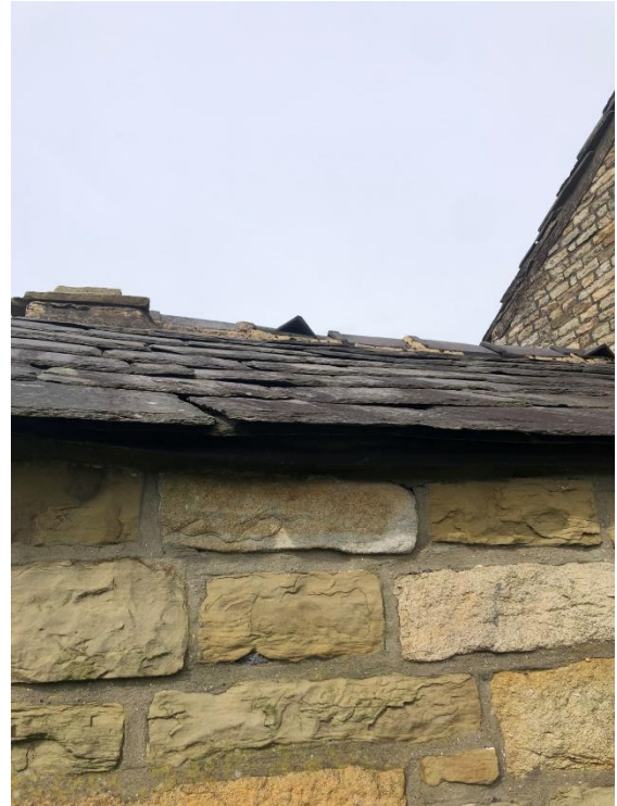
Photograph 7: Welsh slate roof on outbuilding with gaps allowing access to felt underlay.
