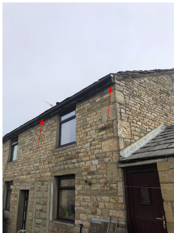
Photograph 3: View of the western elevation with the gap between the stone and fascia board. House sparrows observed entering this gap.
