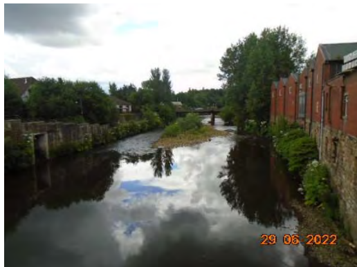
Photo 1: River Irwell. Invasive weeds along the wall of the market
