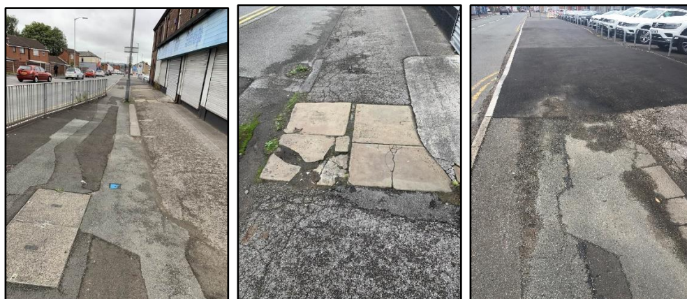
Deteriorated footway in vicinity of new development with evidence of ponding
