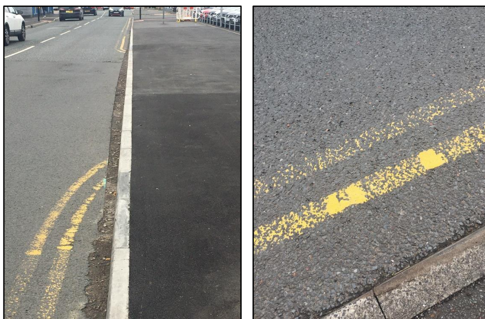
Edge of carriageway not reinstated and double yellow lines incomplete and faded.
