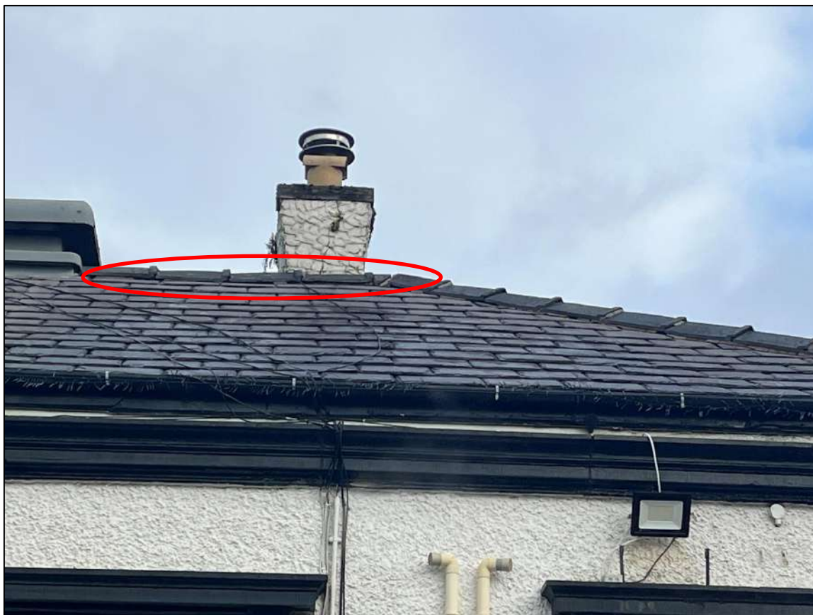
Plate 3 – Examples of PRFs along ridge of clubhouse
