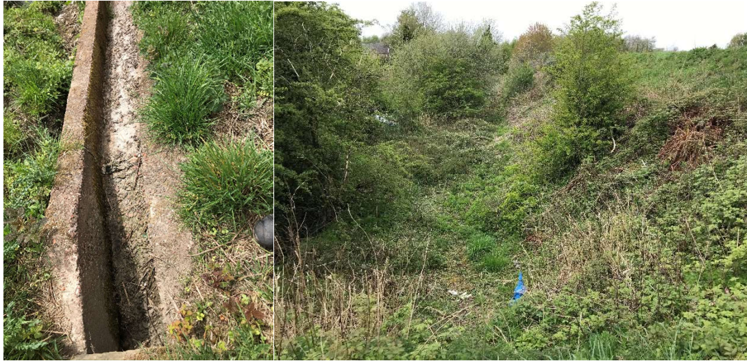
Photographs 1 and 2 – showing the high-level overflow and low-level drain-down valve
