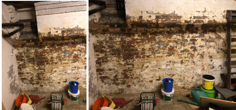
Image 04: existing water egress damage (in basement area)
