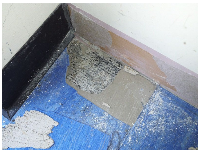
Sample No: Refer to Sample 23/5/B/18/SAW1 G.05 Rear circulation Floor below screed Bitumen adhesive residuals containing: Chrysotile
