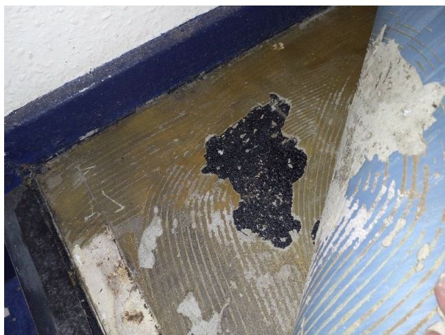
Sample No: 23/5/B/18/SAW5 1.01 Landing Floor below screed Bitumen adhesive residuals containing: Chrysotile
