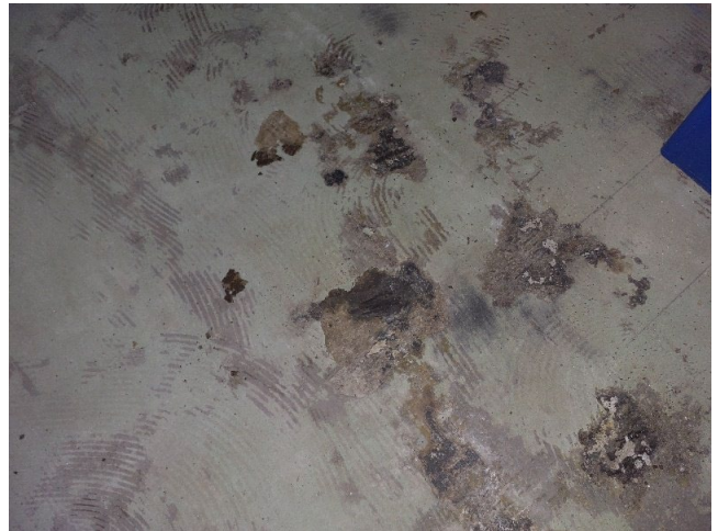
Sample No: 23/5/B/18/SAW1 G.01 Shop area Floor below screed Bitumen adhesive residuals containing: Chrysotile
