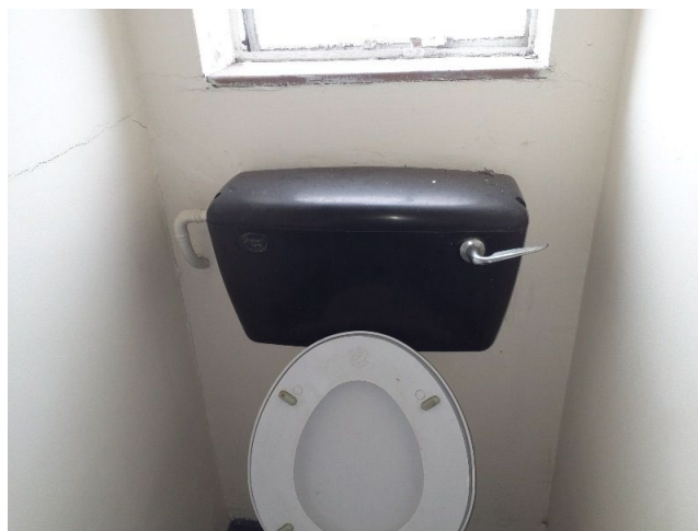
Sample No: 23/5/B/18/SAW9 2.03 Toilet Wall Thermoplastic cistern containing: Amosite
