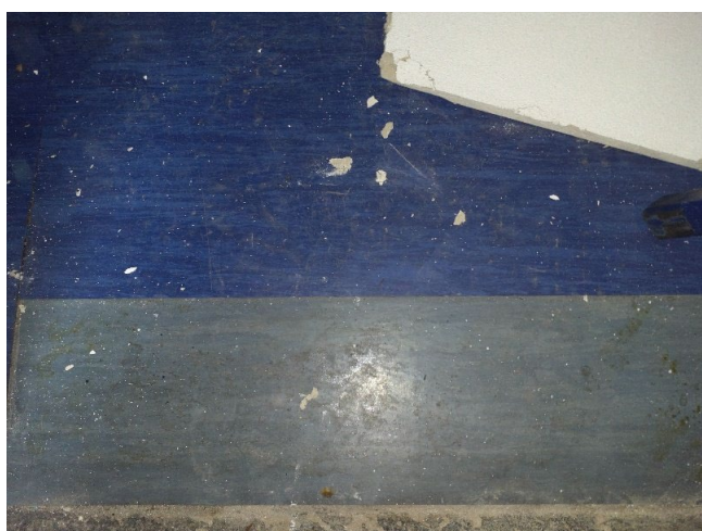
Sample No: Refer to Sample 23/5/B/18/SAW4 1.05 Toilet and lobby Bottom layer of floor covering Vinyl floor covering No Asbestos Detected
