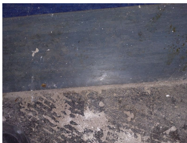
Sample No: Refer to Sample 23/5/B/18/SAW5 1.05 Toilet and lobby Floor below screed Bitumen adhesive residuals containing: Chrysotile
