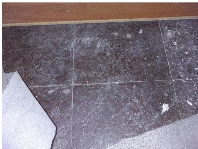
Sample No: 23/5/B/18/SAW15 1.01 Landing Floor Vinyl floor tiles with bitumen adhesive containing: Chrysotile (In both tile and bitumen)
